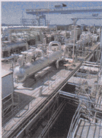
Power equipment checked out in start-up campaign.
