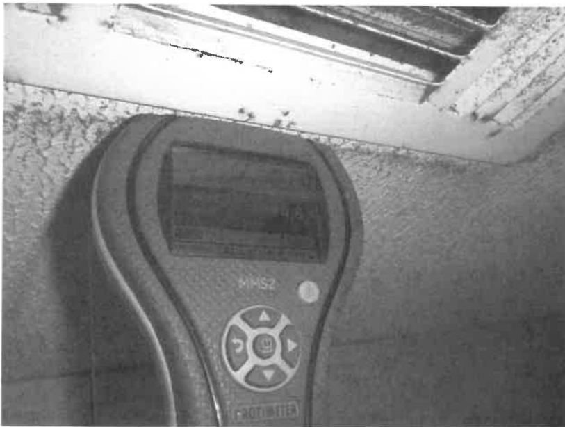
Photo 6. Elevated moisture level of 24.8% in ceiling material next to AC vent in men's restroom
