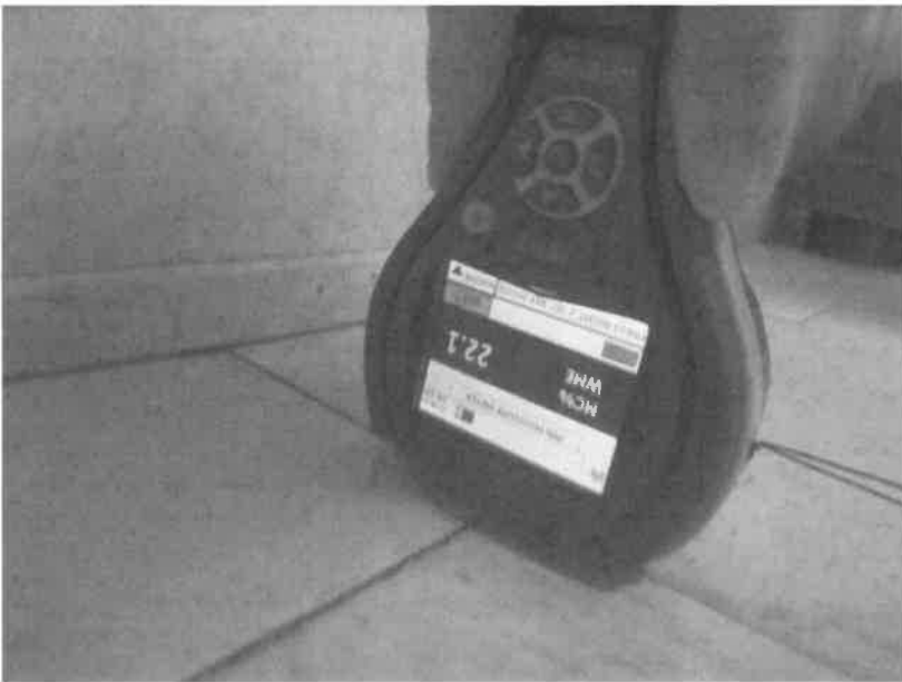
Photo 19. Elevated moisture level in floor of women's restroom
