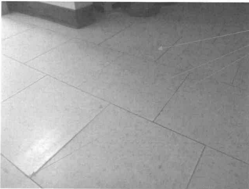
Photo 10. Damaged flooring outside of storage room
