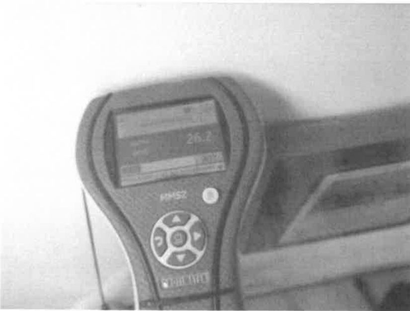
Photo 14. Elevated moisture level in south wall of conference room a few feet down from vent
