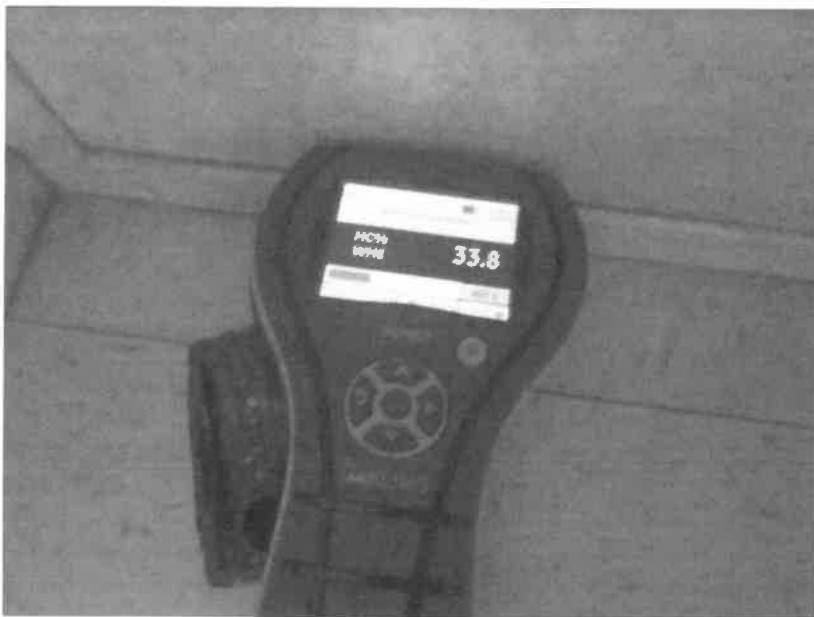
Photo 7. Elevated moisture level in base of west wall of men's restroom
