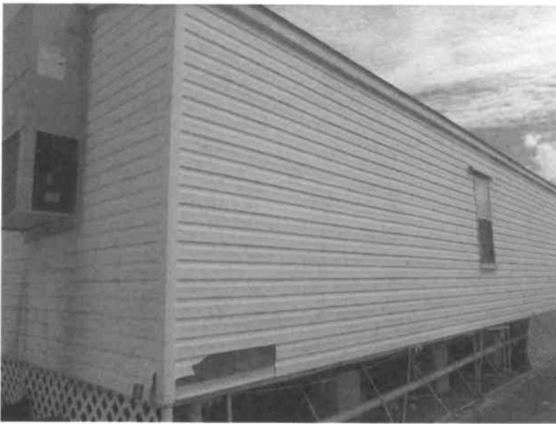
Photo 25. Damage to siding on west side of building
