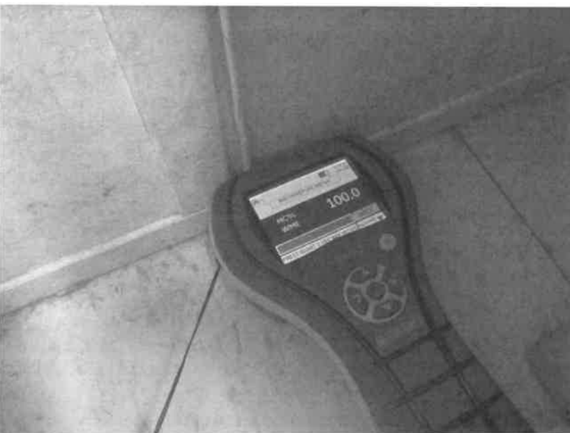
Photo 15. Elevated moisture level in base of wall under window on east wall just outside of women's restroom
