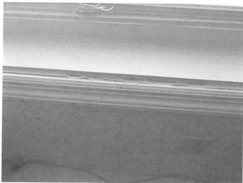
Photo 24. Damage to window frame in Kaitlin's office
