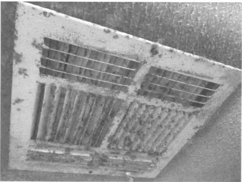
Photo 8. Air conditioning vent with fungal growth in Lab
