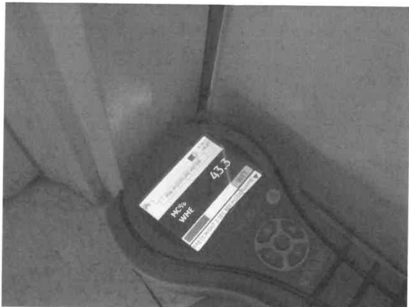
Photo 22. Elevated moisture level in left side of door frame to door outside of Kaitlin's office
