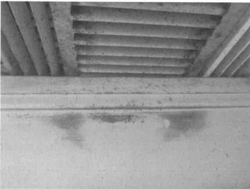
Photo 12. Vent and adjacent wall with fungal growth in conference room
