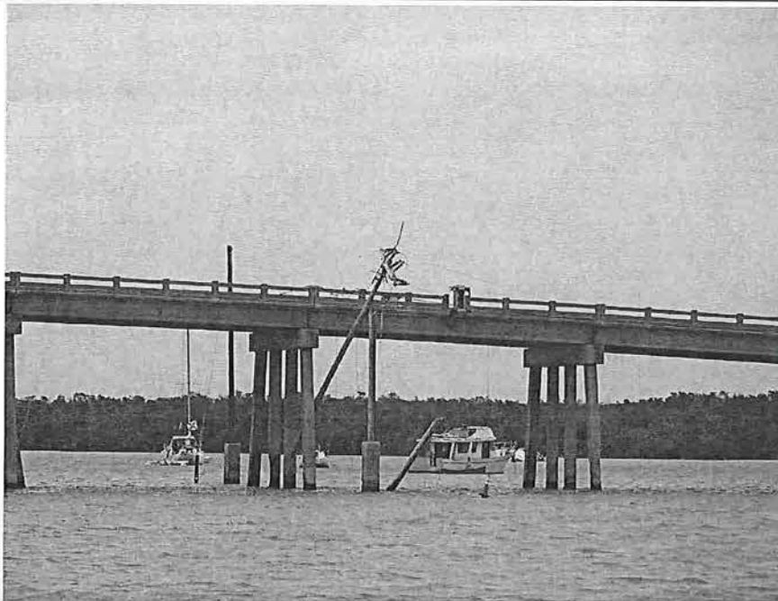
20TH STREET BRIDGE WHERE BROKEN POWER LINE POST IS VISIBLE
