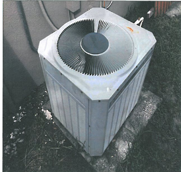
The condenser was manufactured in 1989.
