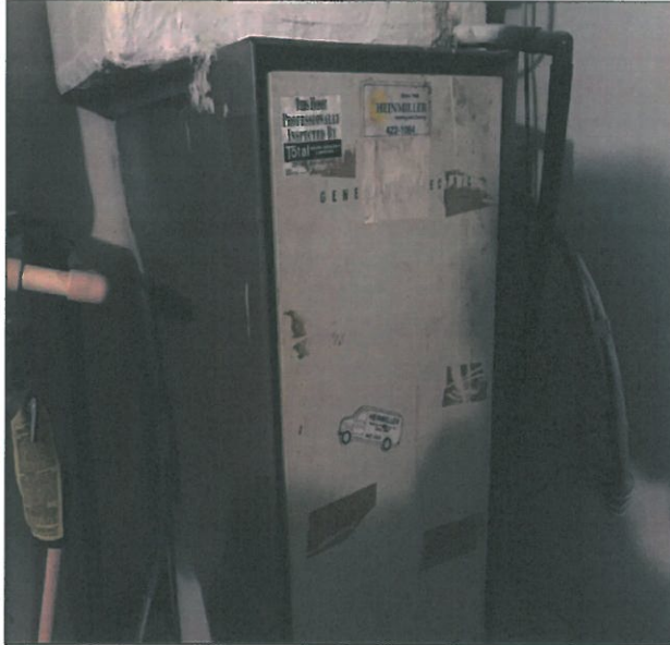
Possibly the original air handler (1973).
