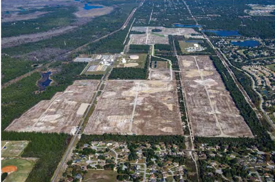
FIGURE 3.8 DeBary Solar Site
