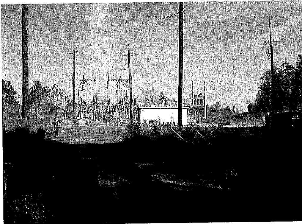
Photograph 20 – View to the north showing the Florida Power and Light Substation adjoining to the north of the northeastern portion of the property.
