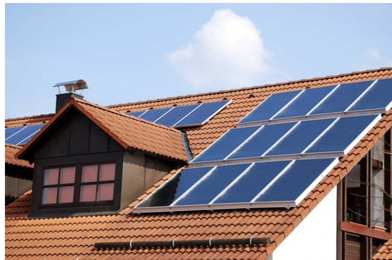
House roof with solar panels.
