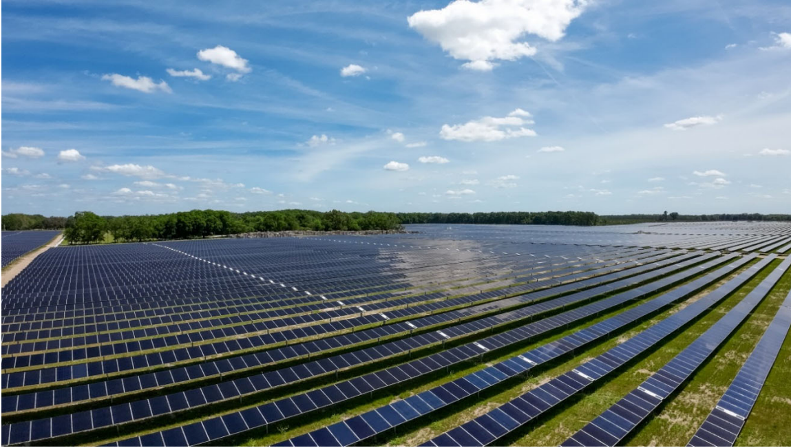
FIGURE 3.4 High Springs Solar Power Plant
