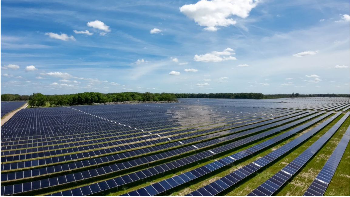
FIGURE 3.4 High Springs Solar Power Plant
