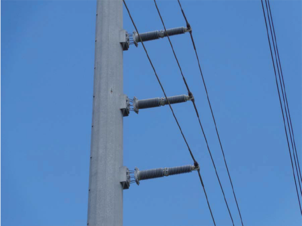
Steel pole AFC-6 post insulator hardware damage. Looking north.
