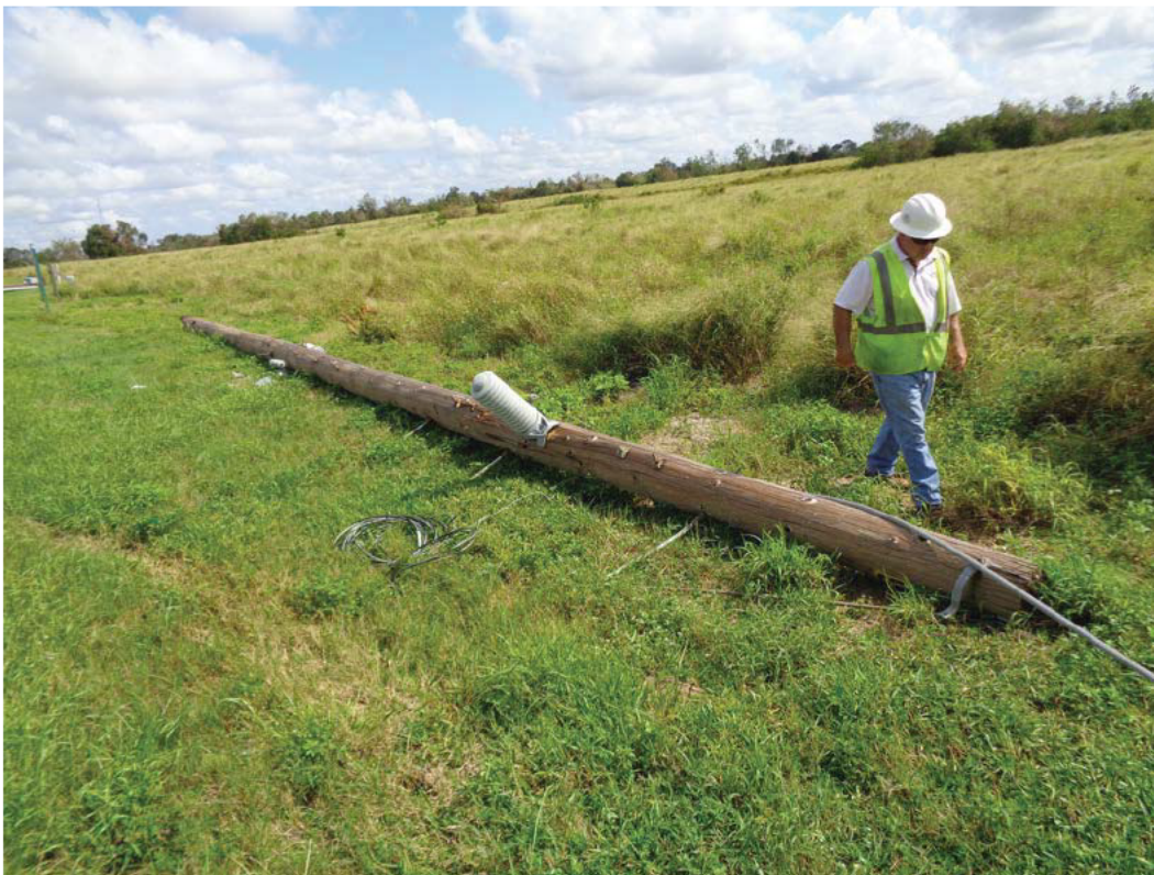
Failed wood pole AD-19. Looking northeast.
