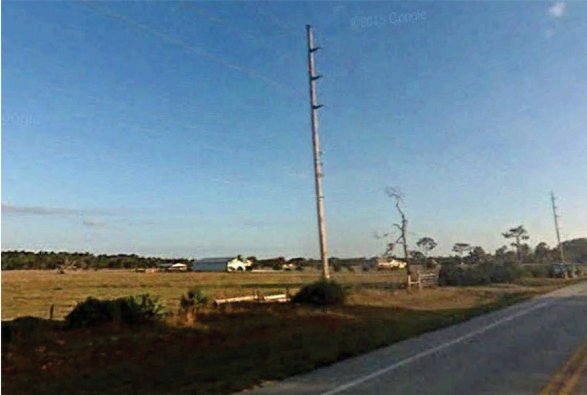
Figure 15: Failed pole ALP-225, looking southeast.
