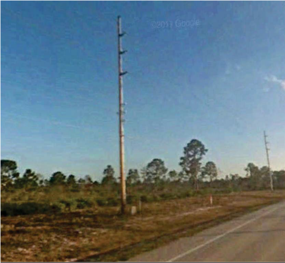
Figure 10: Failed pole ALP-206, looking southeast.
