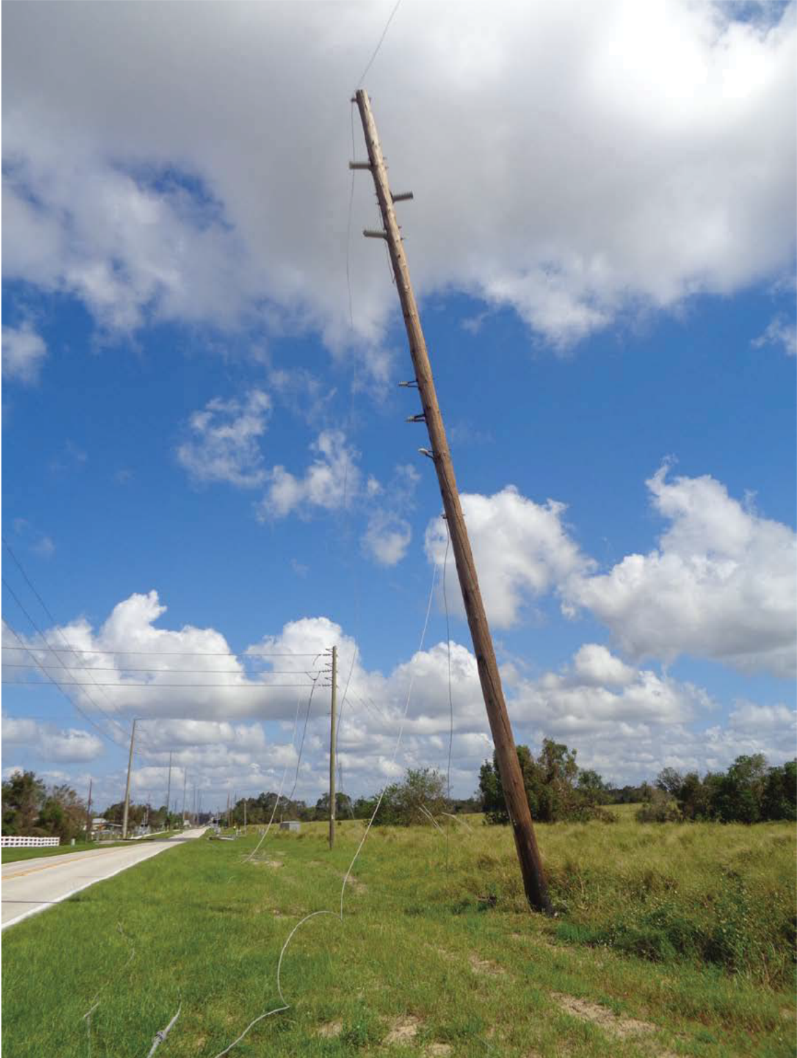
Damaged wood pole AD-17. Looking north.
