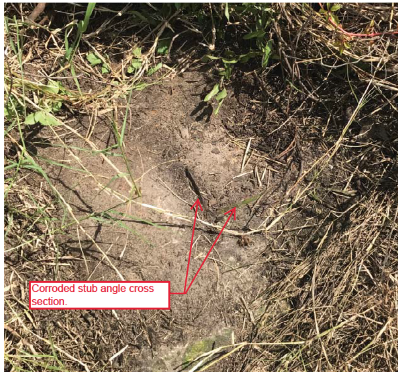
HG-160 NW foundation, corroded-sheared stub angle.
