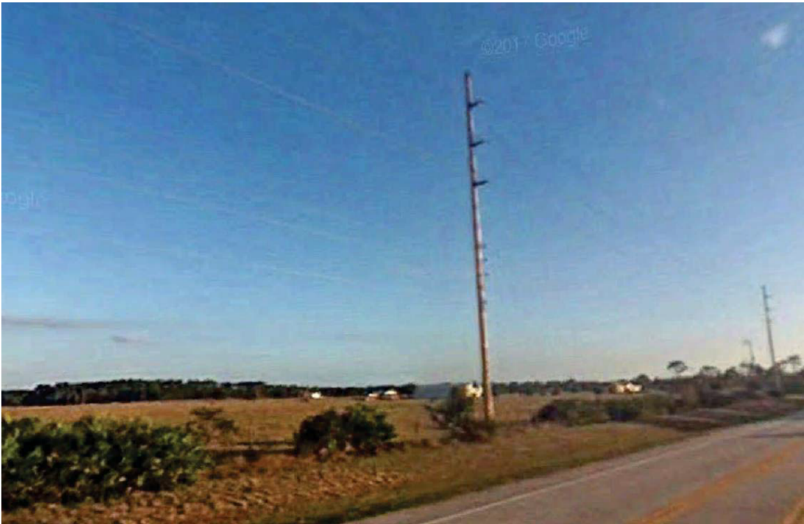
Figure 14: Failed pole ALP-224, looking southeast.
