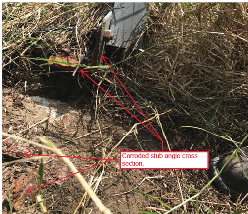
HG-160 SW foundation, corroded-sheared stub angle.
