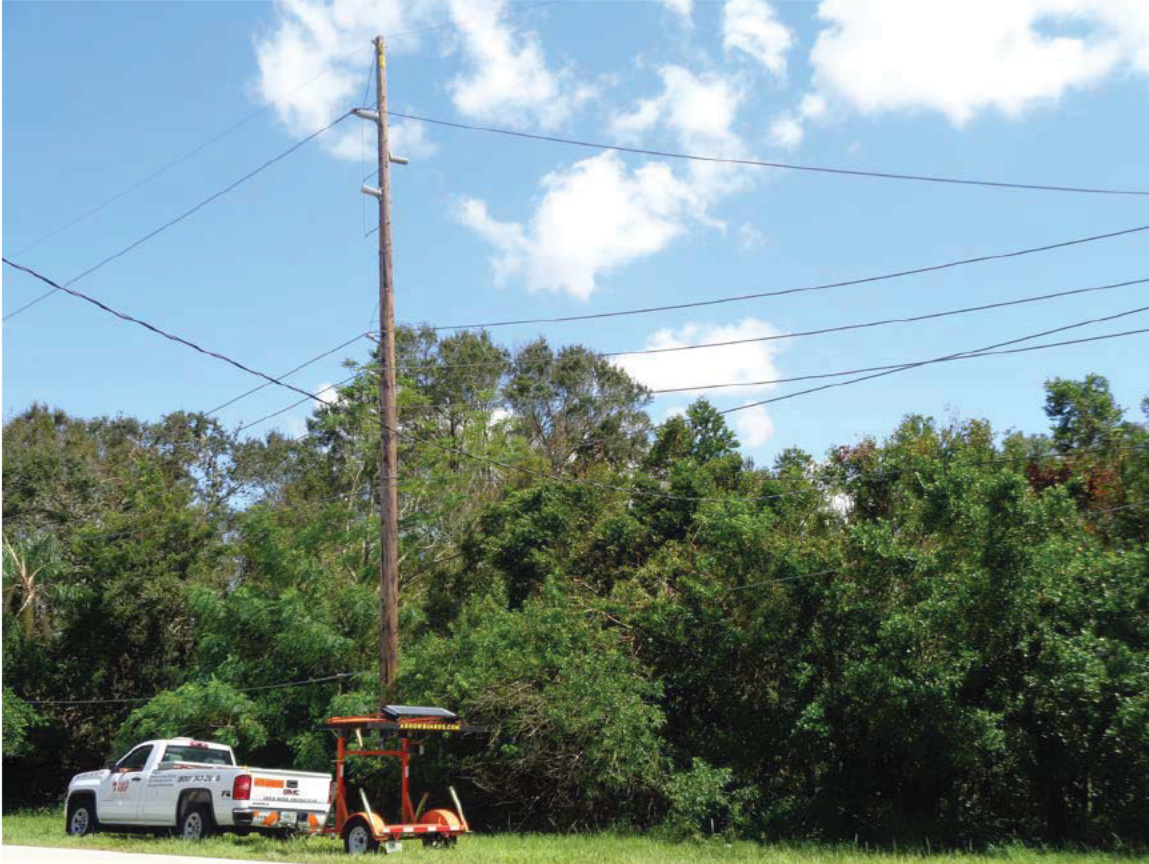
Wood pole AD-10 post insulator damage. Looking east.
