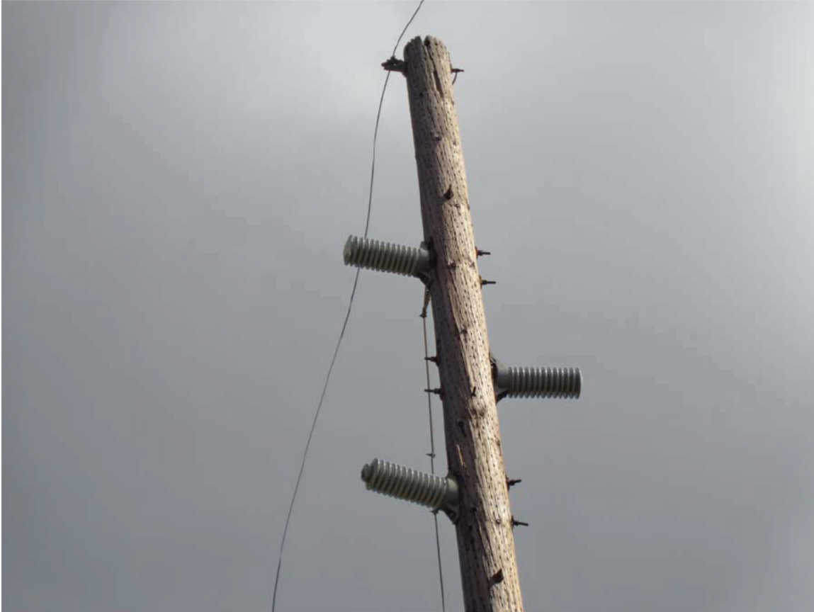
Wood pole AD-17 insulator damage. Looking north.
