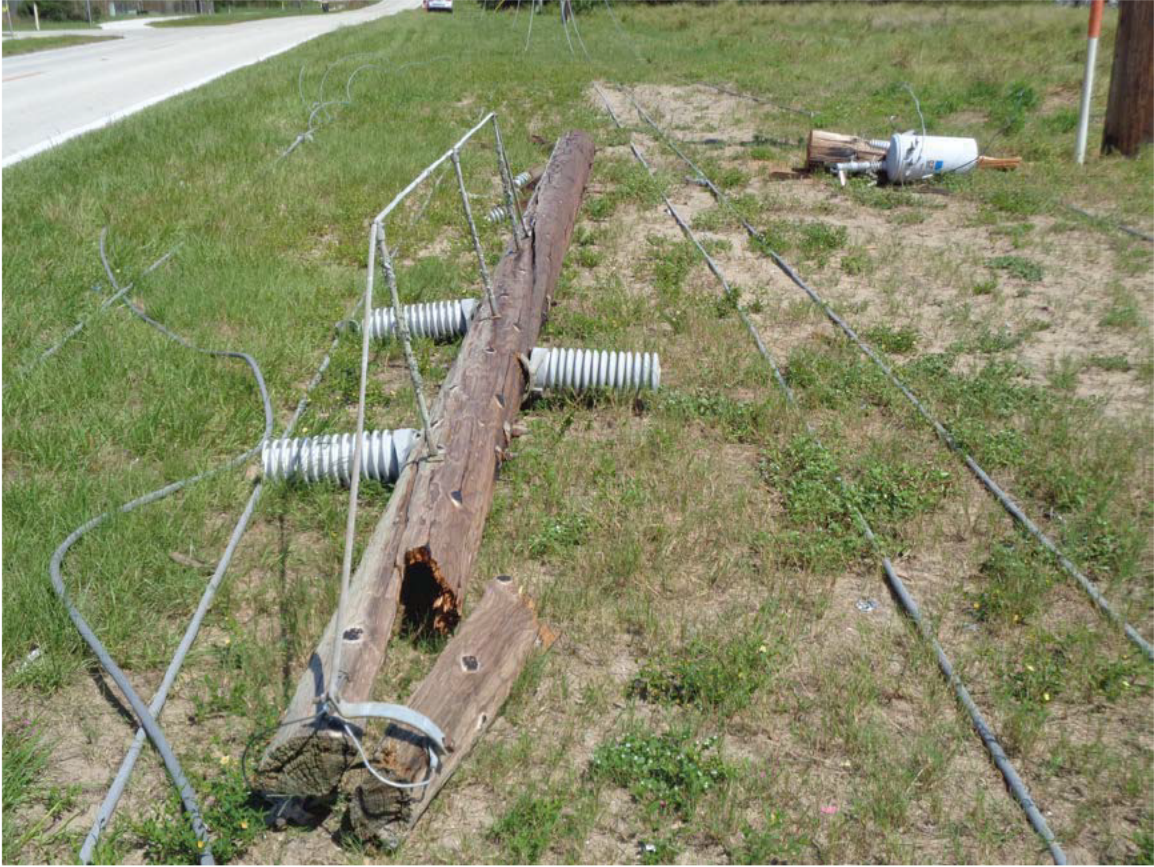
Failed wood pole AD-12. Looking north.
