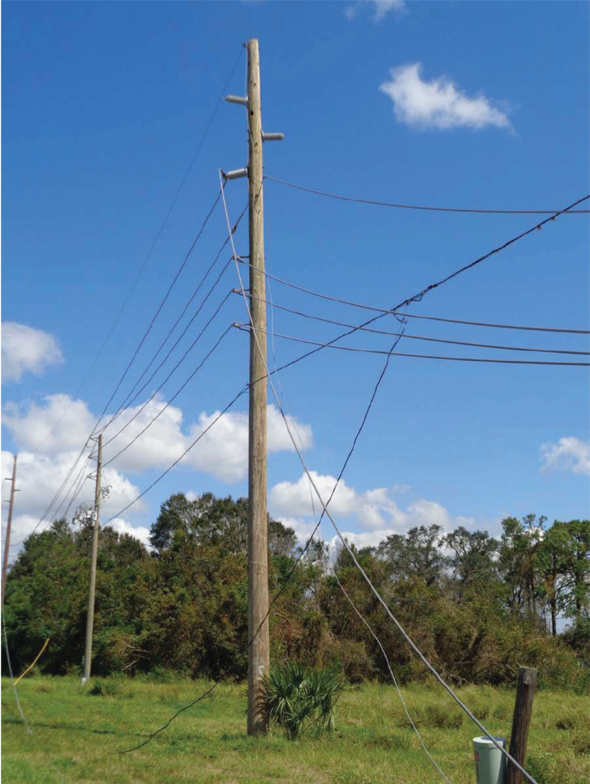
Wood pole AD-11 post insulator damage. Looking east.
