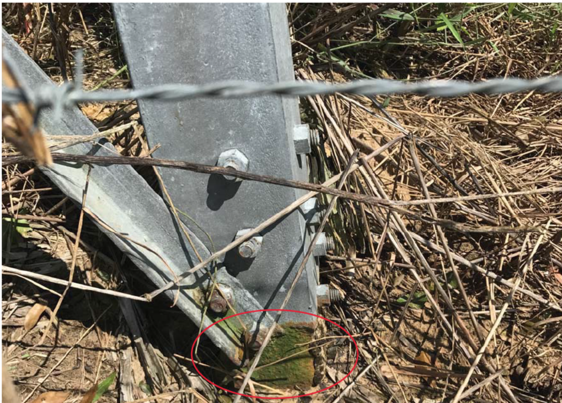
HG-162 SW Leg Corrosion on Stub Angle at Foundation
