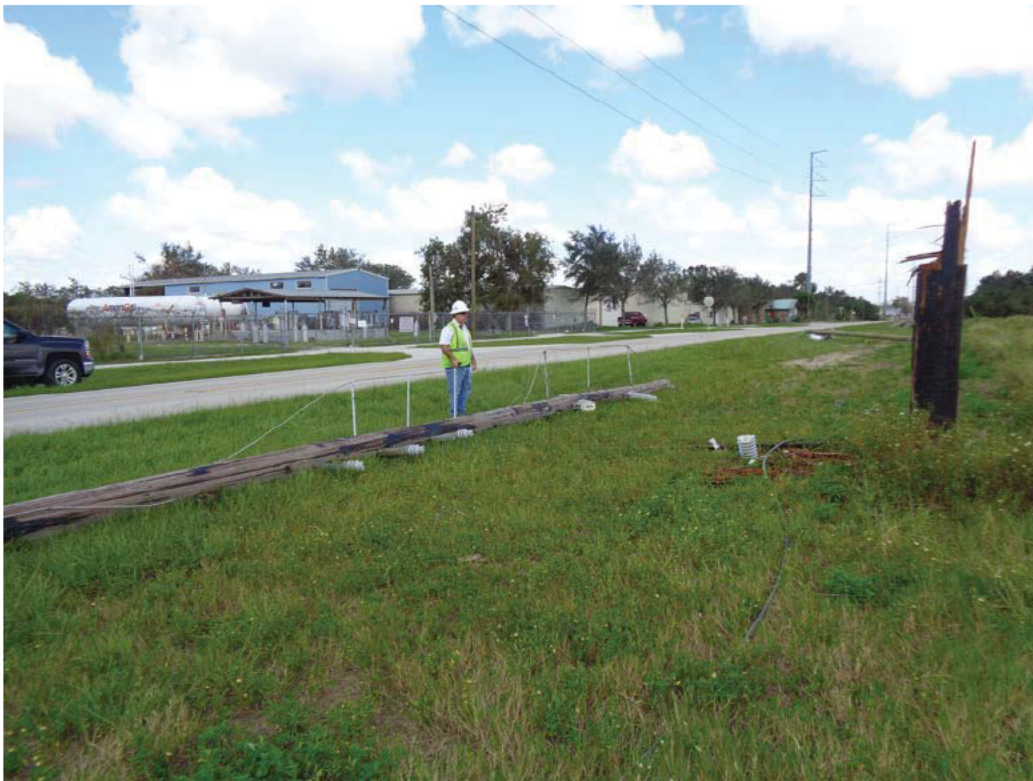
Failed wood pole AD-14. Looking northwest.
