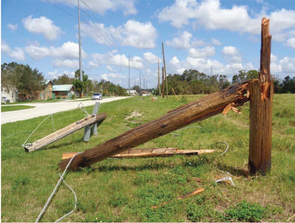
Failed wood pole AD-13. Looking north.
