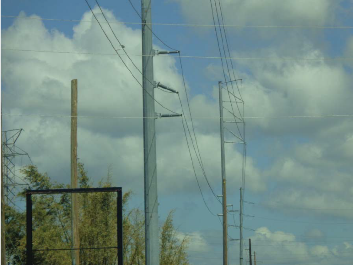
Steel pole AFC-7 post insulator hardware damage. Looking north.
