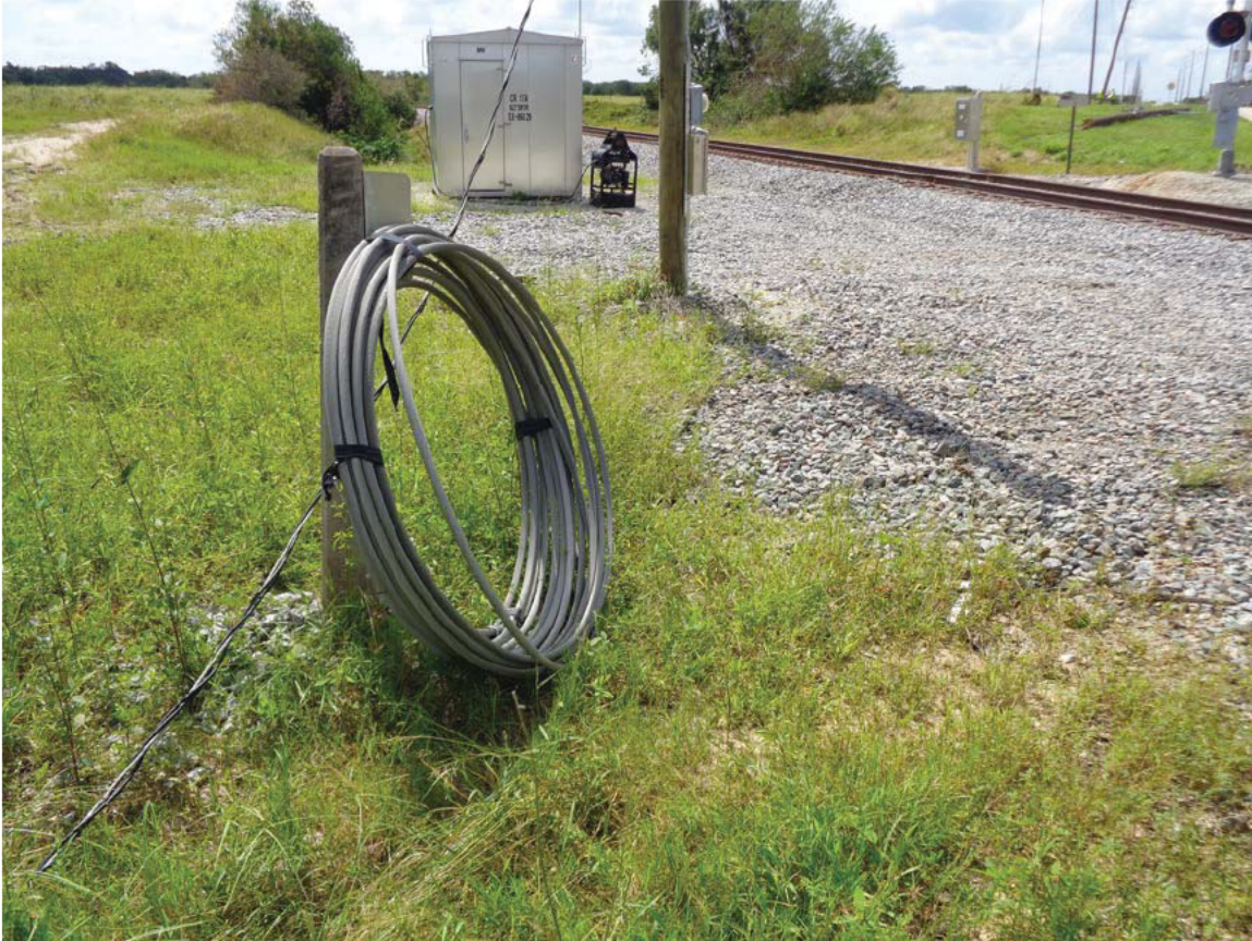
Cut and coiled wire near railroad ROW.
