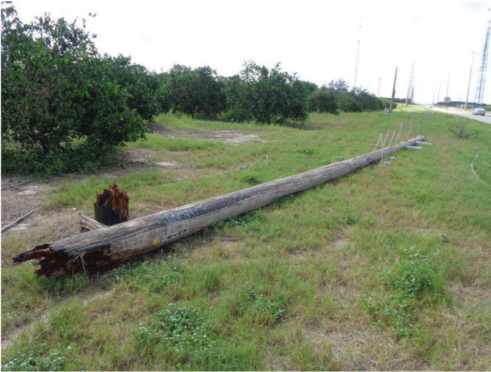
Failed wood pole AD-20. Looking south.
