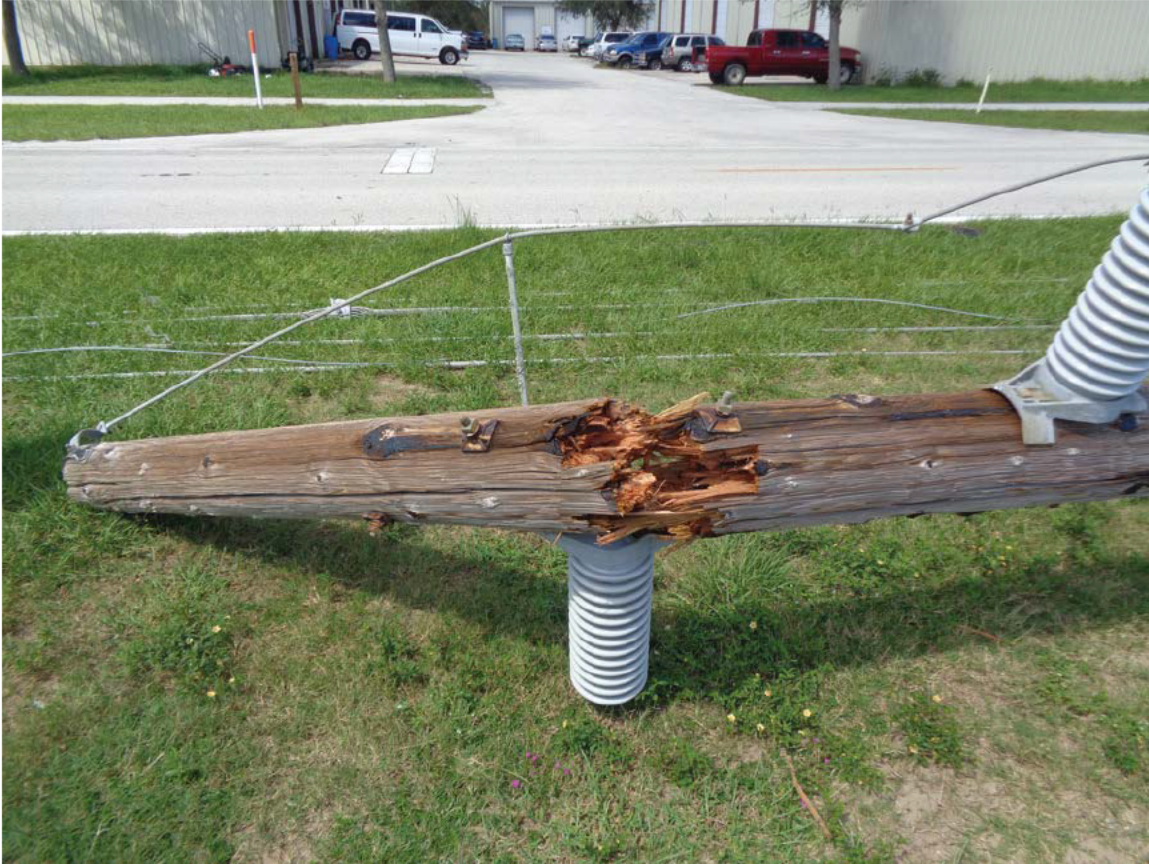
Wood pole AD-13 insulators and wood pole crack. Looking west.
