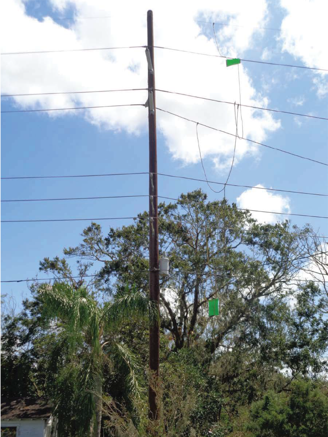
Wood pole AD-9 post insulator hardware damage. Looking east.
