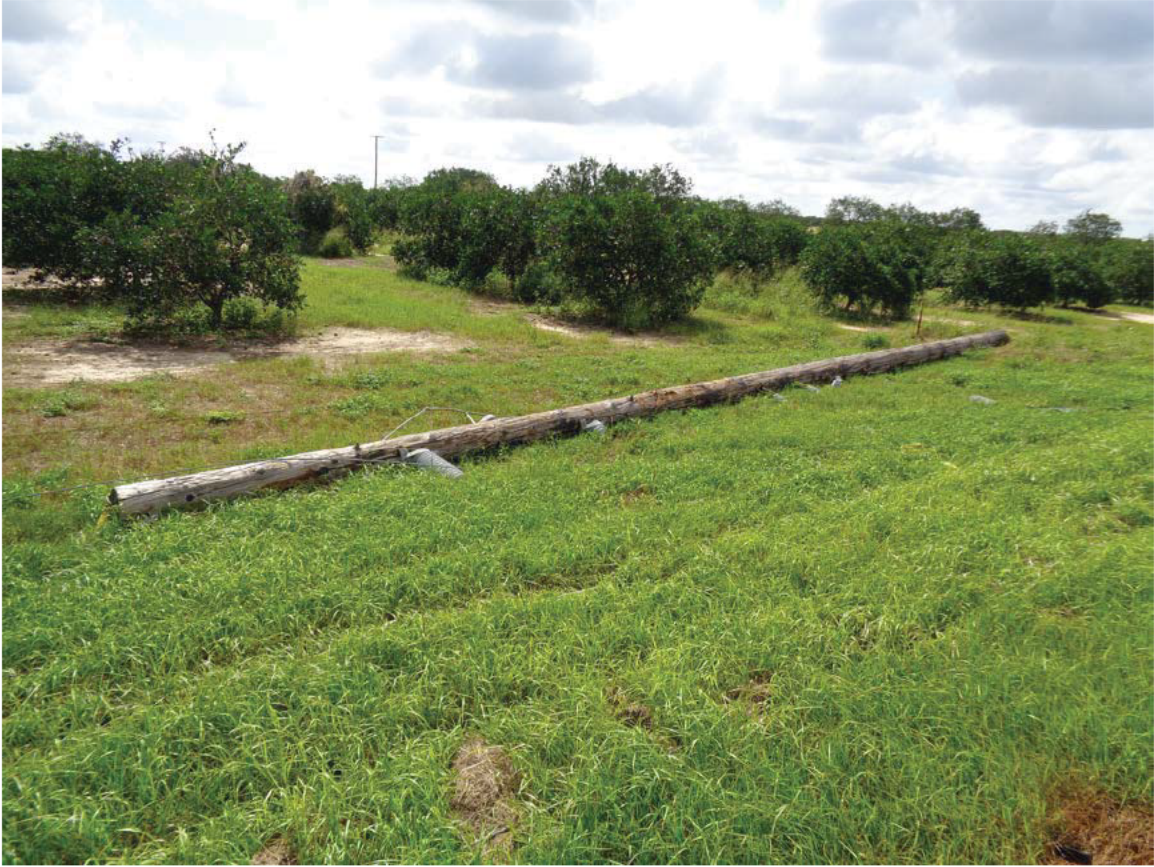
Failed wood pole AD-22. Looking southeast.
