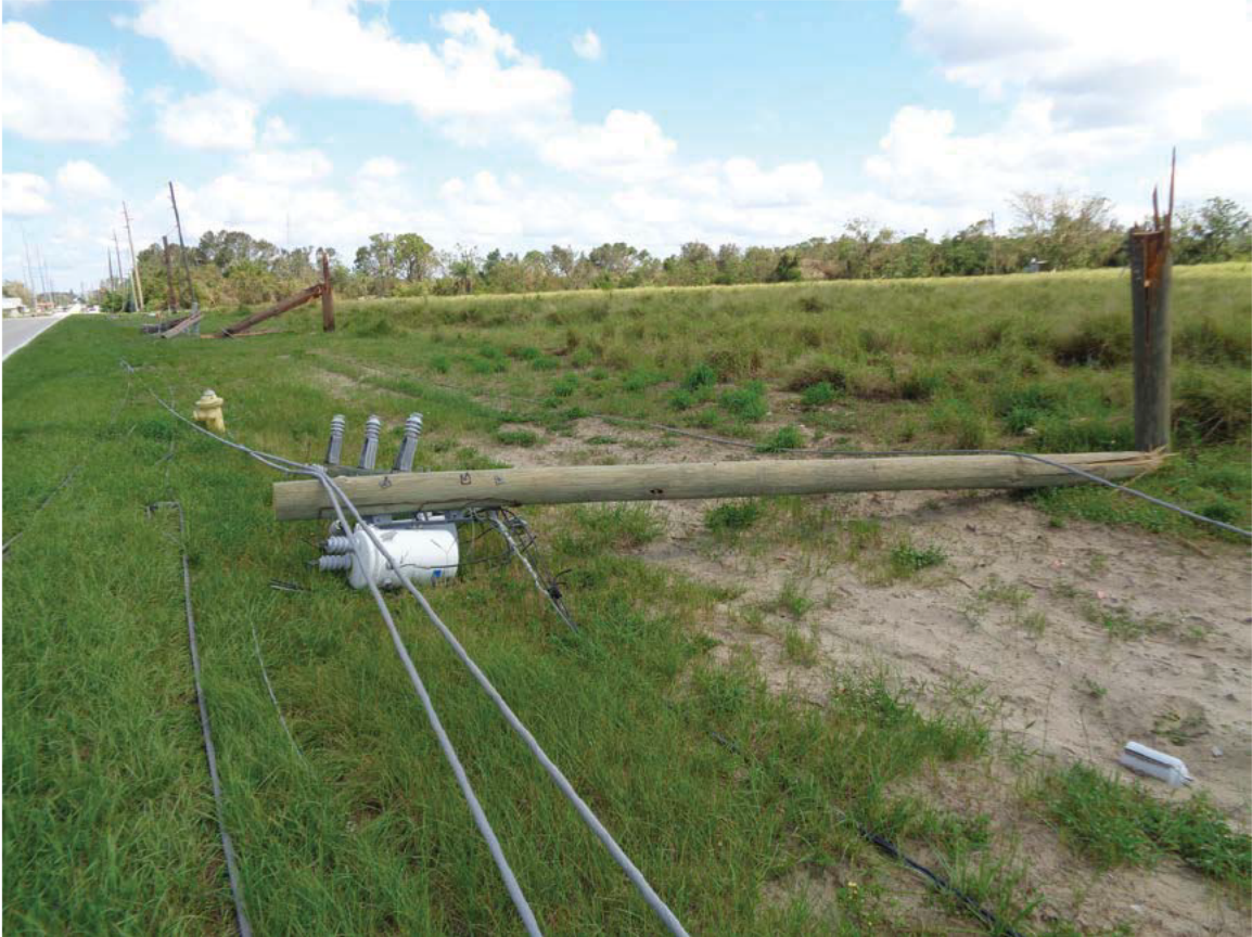
Failed distribution mid span pole. Looking north.
