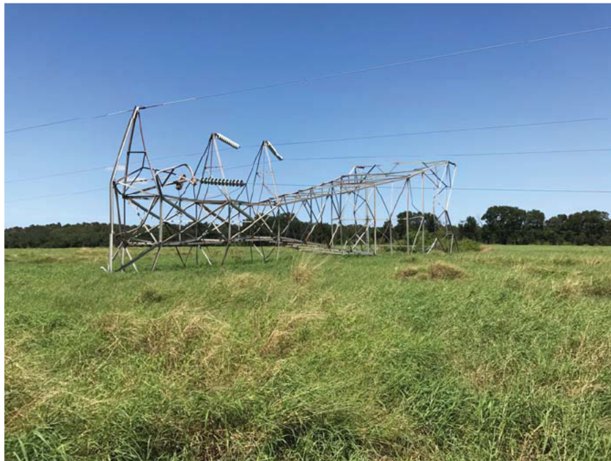
Tower HG-160 failure – Looking Northwest.
