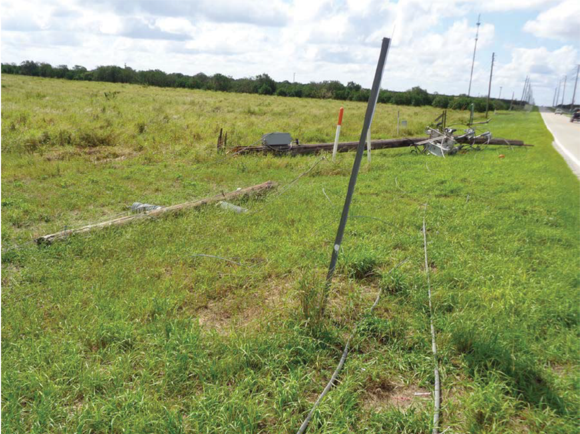
Wood pole AD-18 failure. Pole broke into two. Looking southeast.
