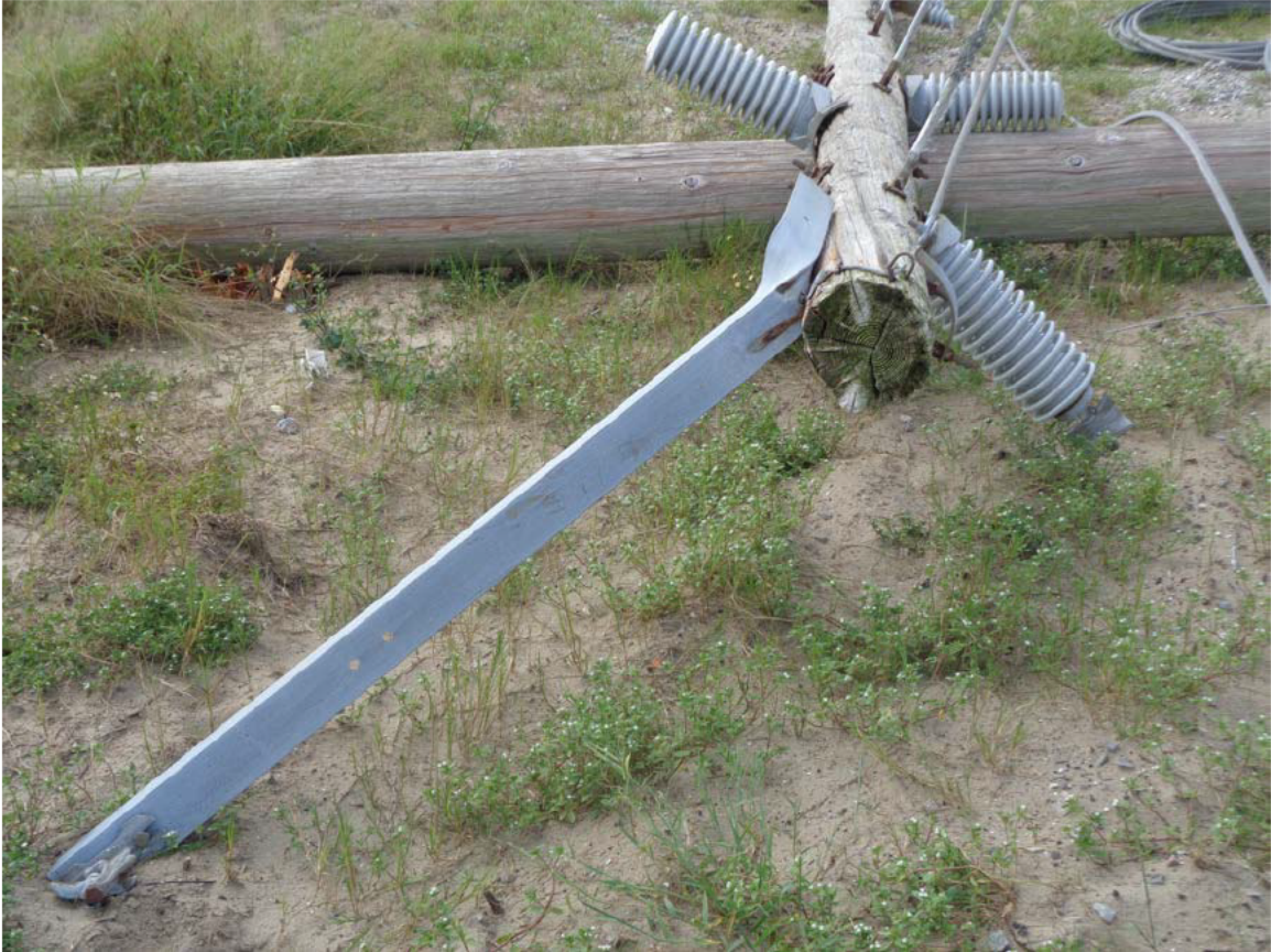
Wood pole AD-15 static mast. Looking south.
