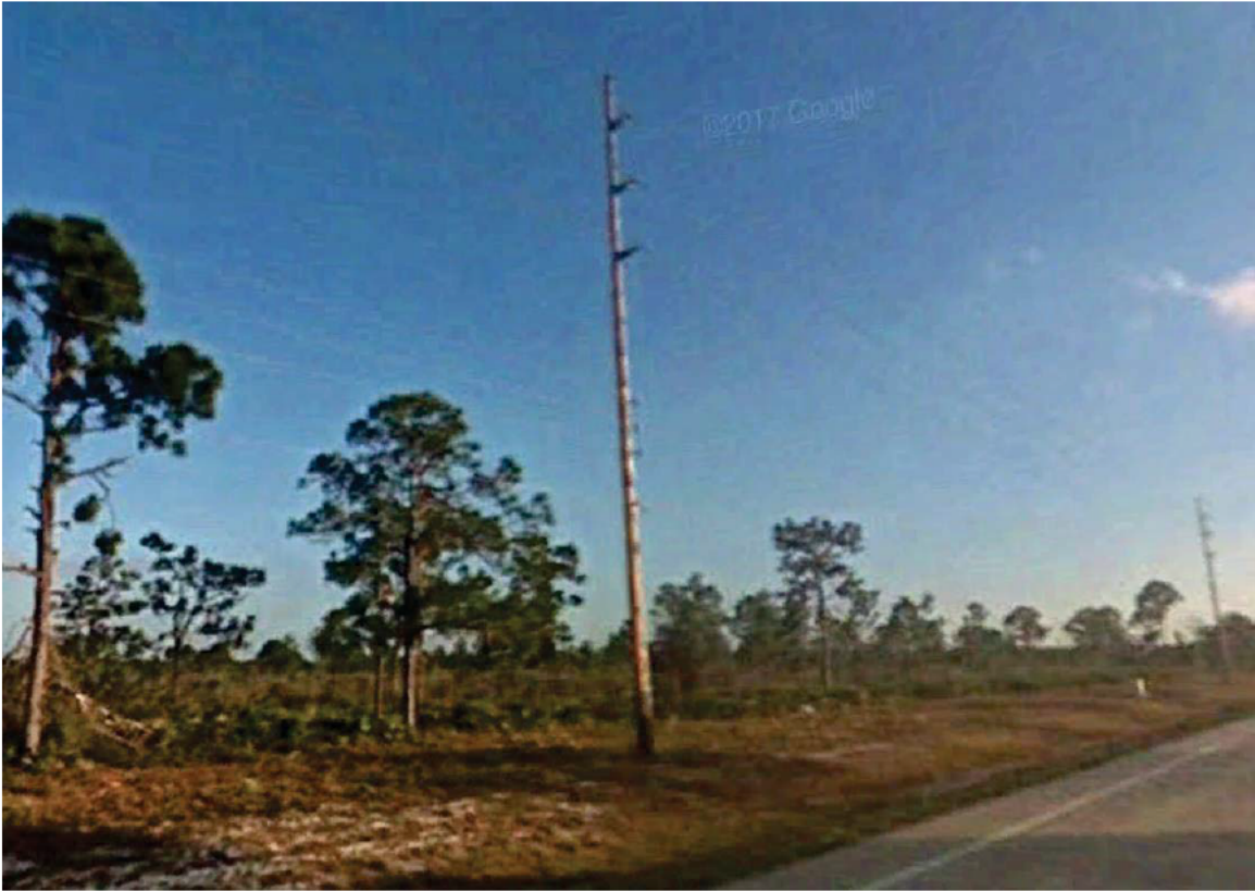
Figure 9: Failed pole ALP-205, looking southeast.
