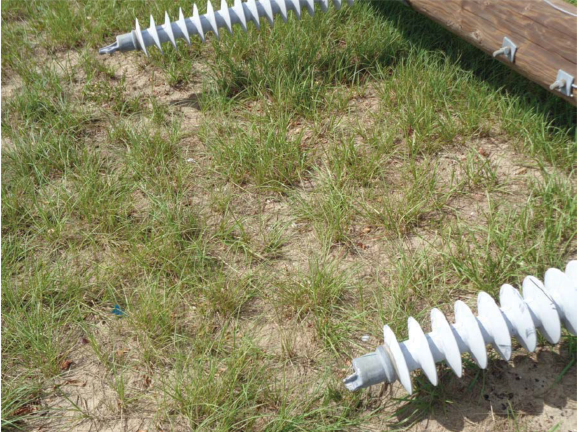
AD-16 post insulator damage. Looking southwest.
