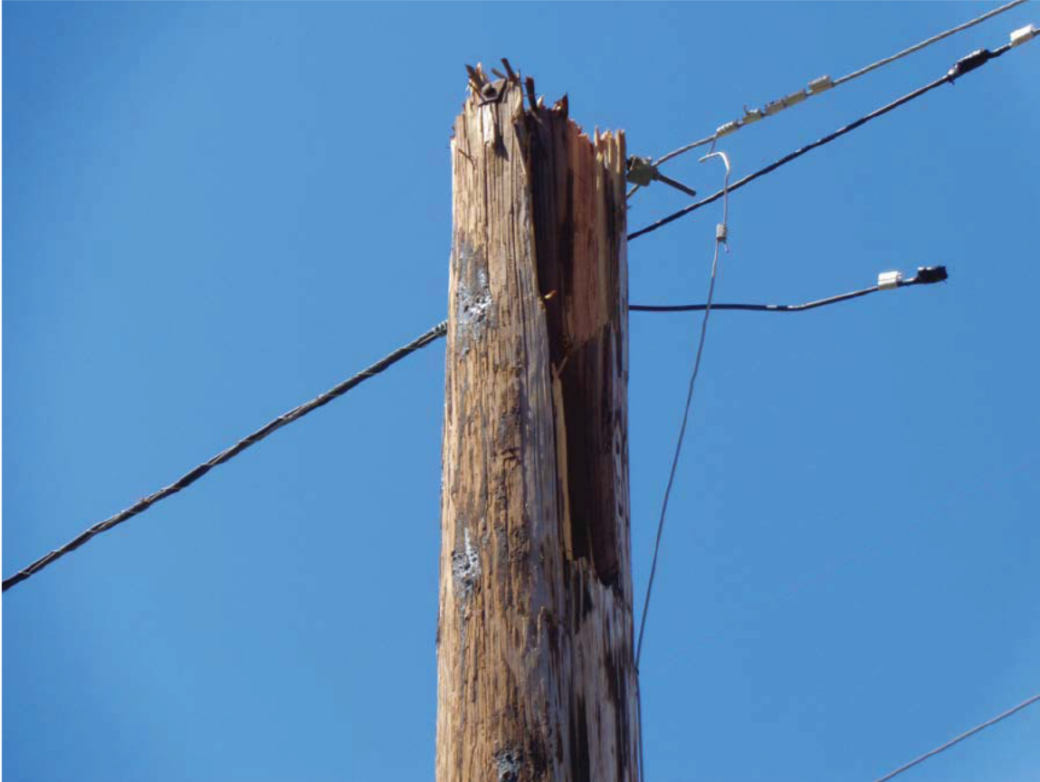
Wood pole AD-12 pole crack. Looking southwest.
