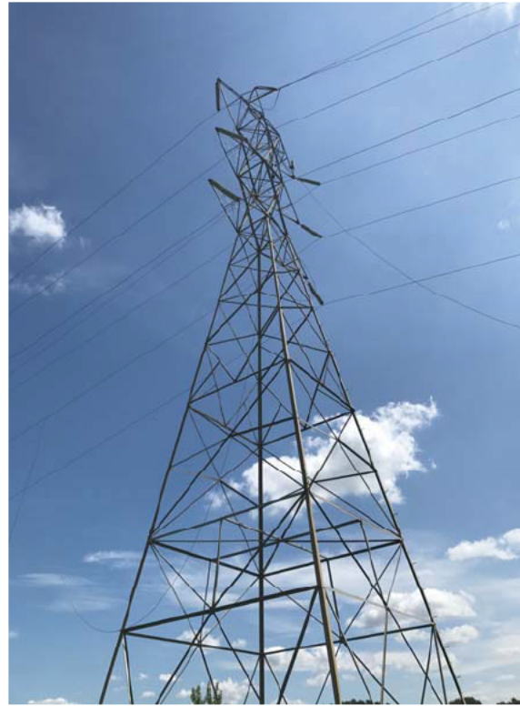
Tower HG-161 damage.
