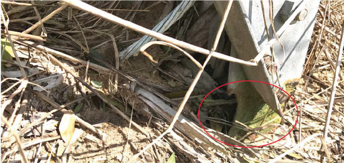
HG-162 Major Section Loss on Stub Angle at Foundation SW Leg
