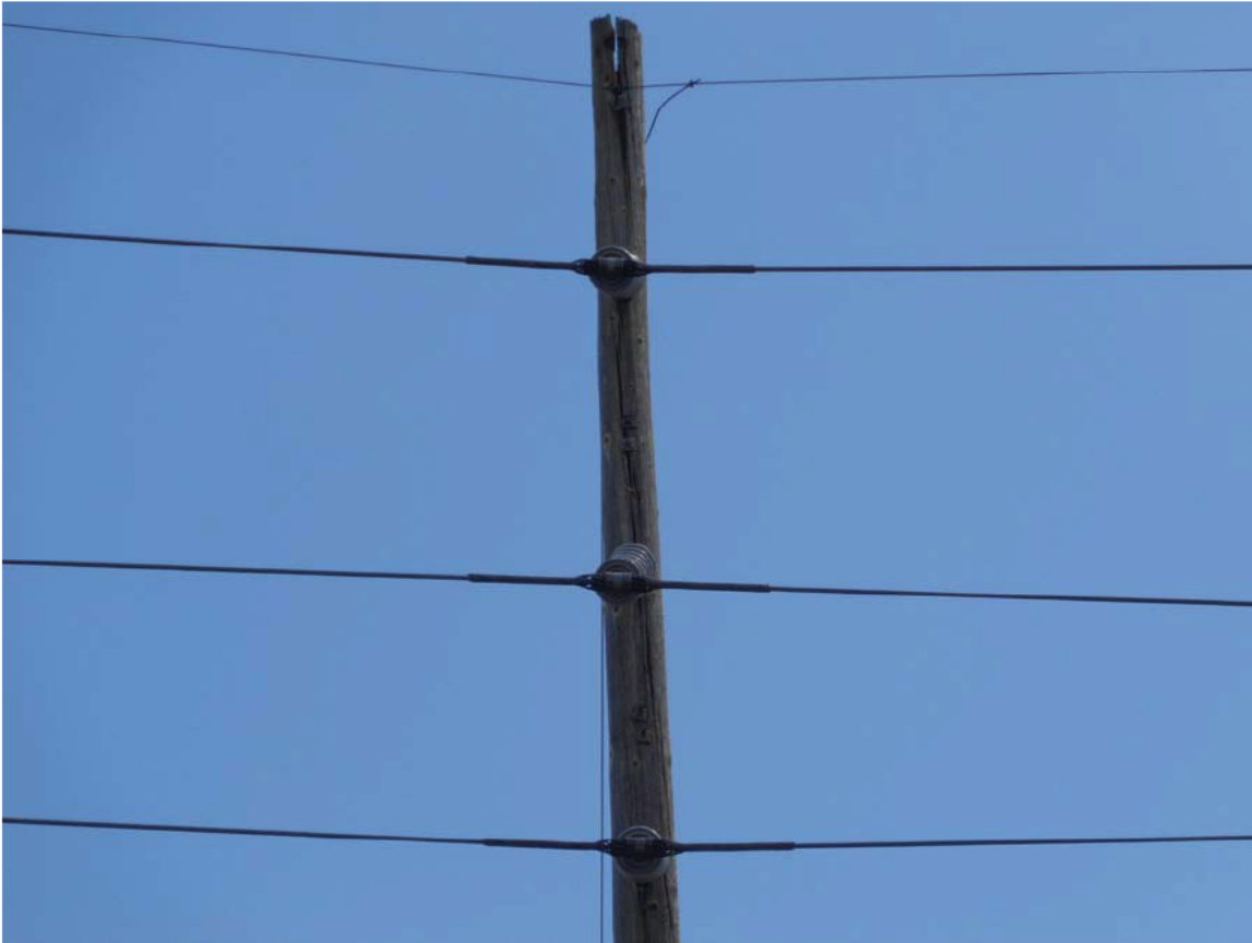
Wood pole AD-8 pole top damage. Looking east.
