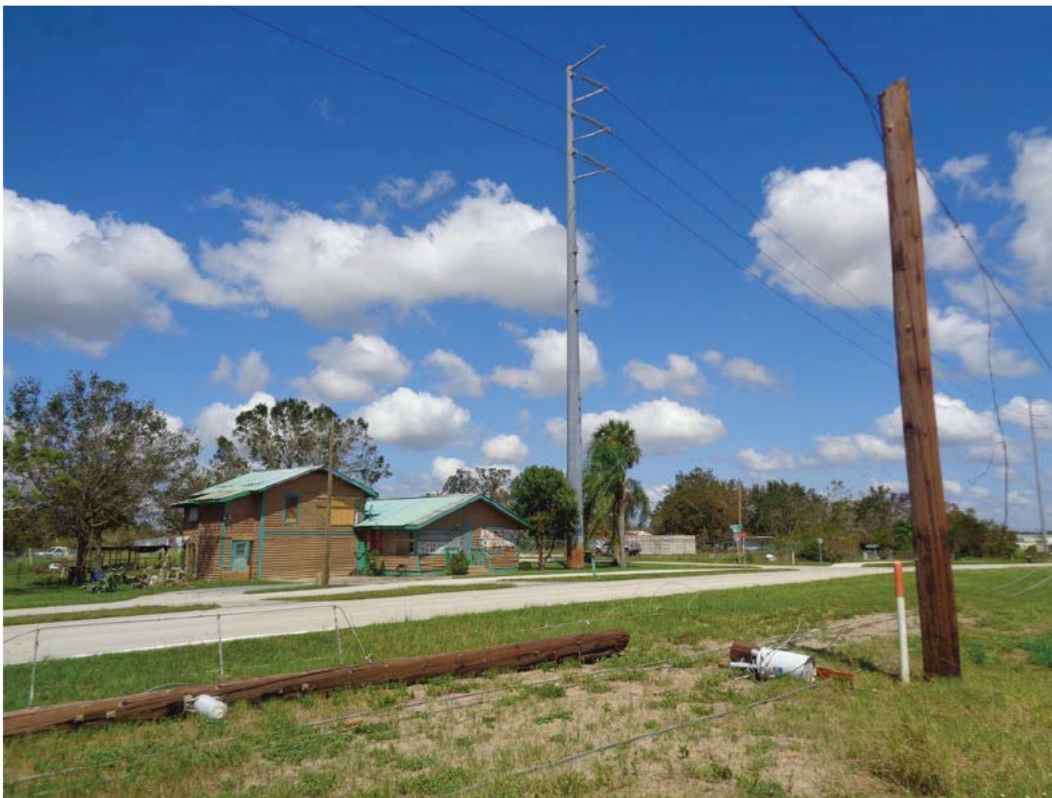
Failed wood pole AD-12. Looking northwest
