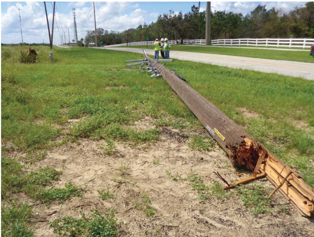
Failed wood pole AD-16. Looking south.
