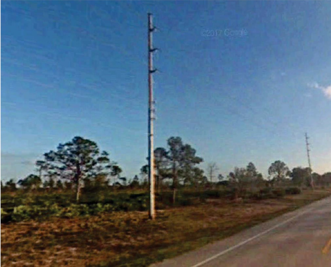
Figure 11: Failed poled ALP-207, looking southeast.
