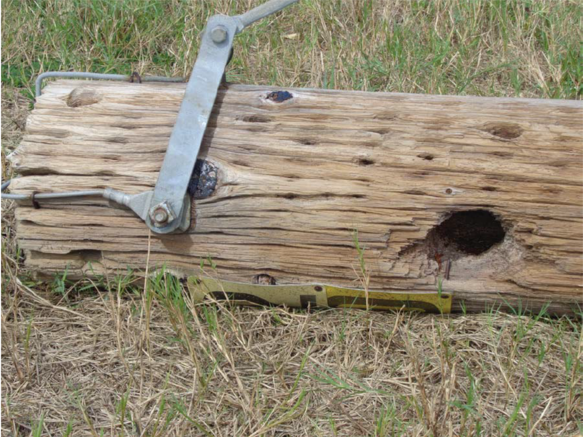
Wood pole AD-20 woodpecker damage. Looking west.
