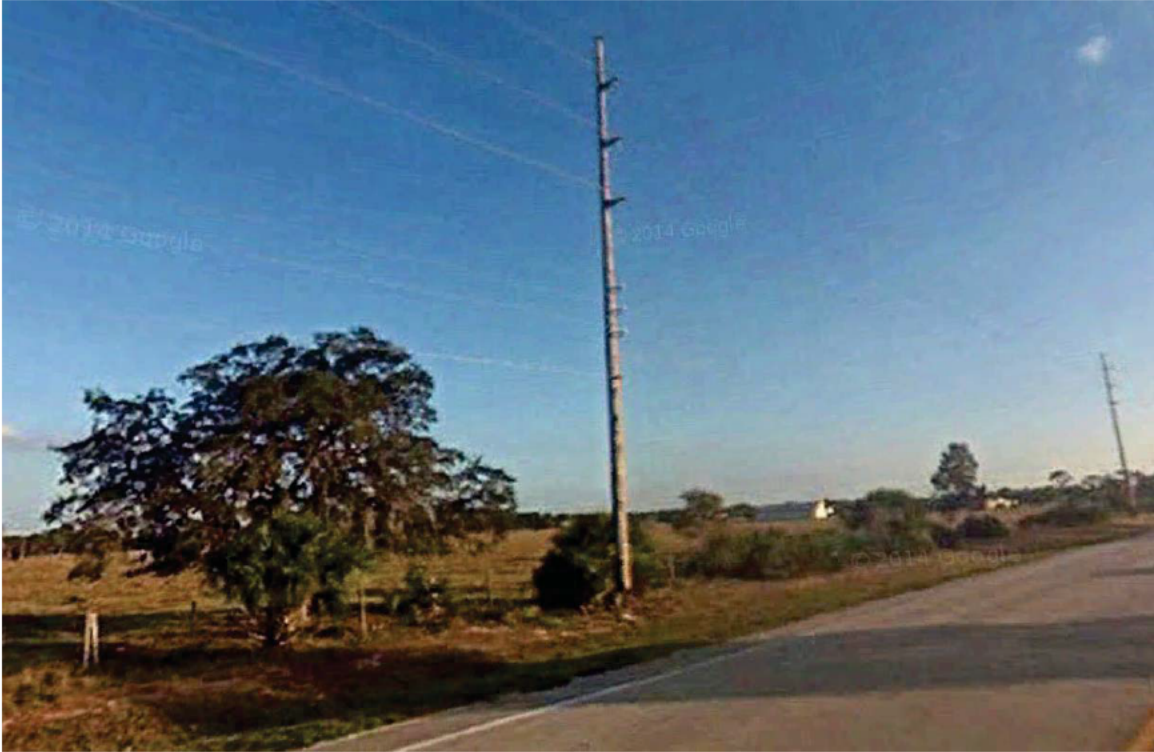
Figure 13: Failed pole ALP-223, looking southeast.
