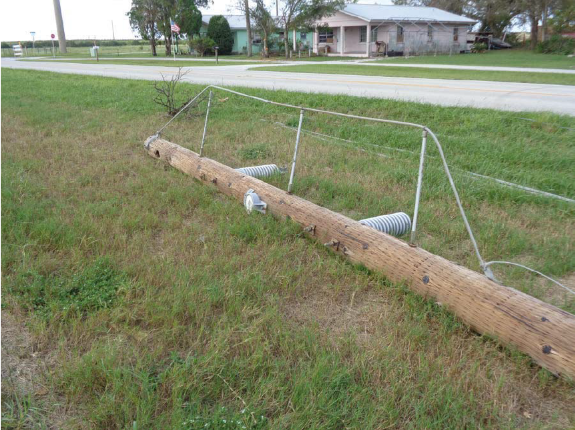
Wood pole AD-20 insulator damage. Looking southwest.
