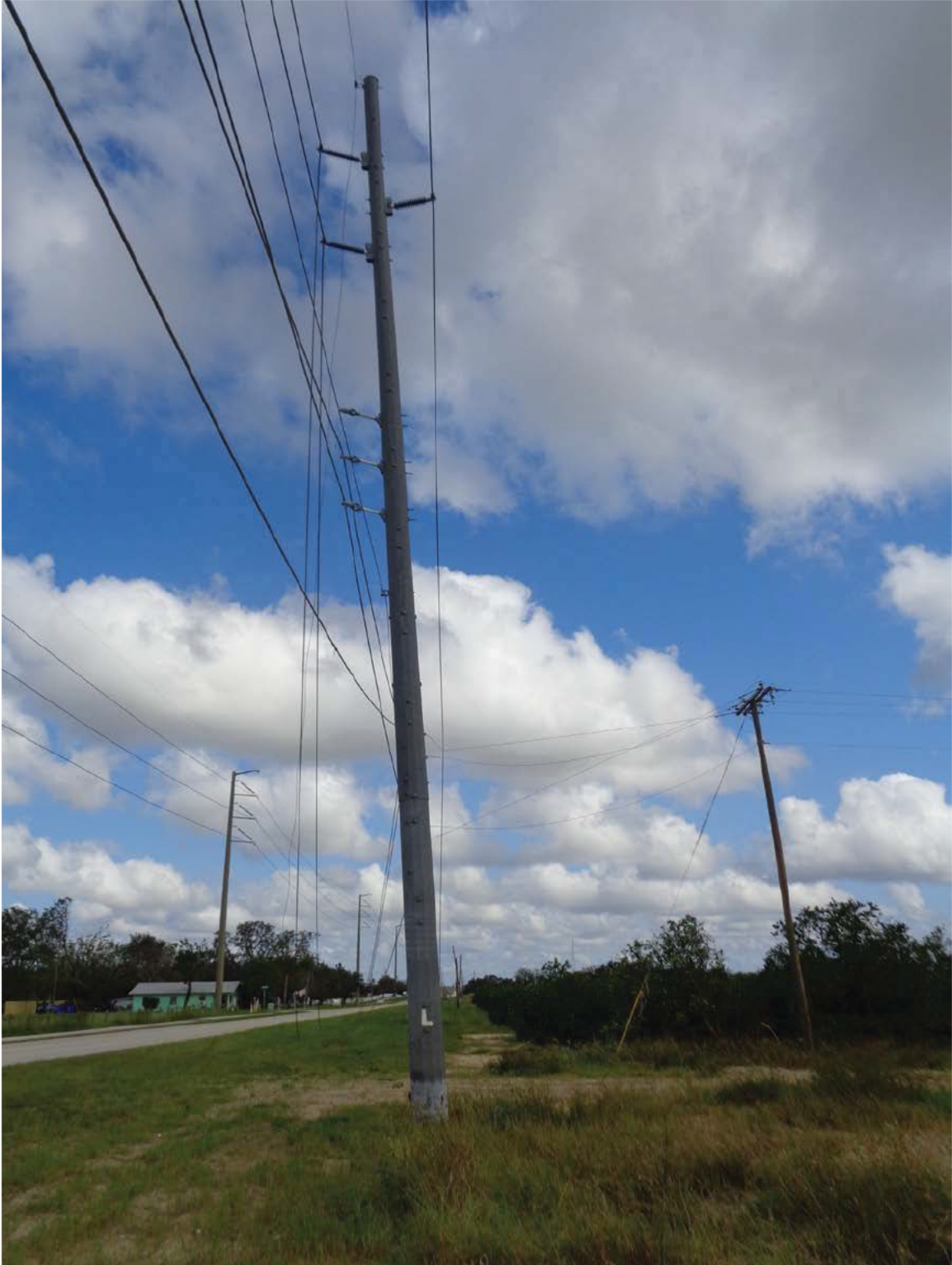
Leaning steel pole AD-23. Looking north.
