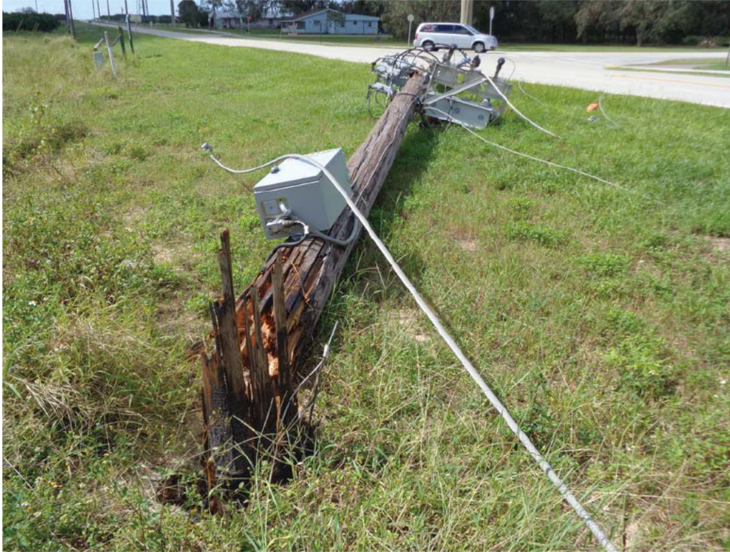
Failed wood pole AD-18. Looking southwest.
