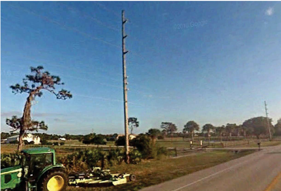
Figure 16: Failed pole ALP-226, looking southeast.
