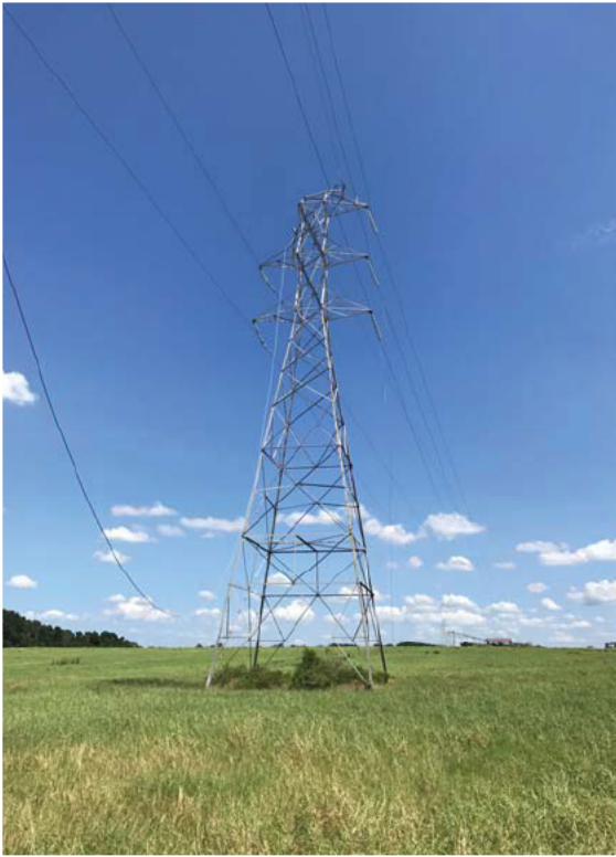
Tower HG-159 damage.
