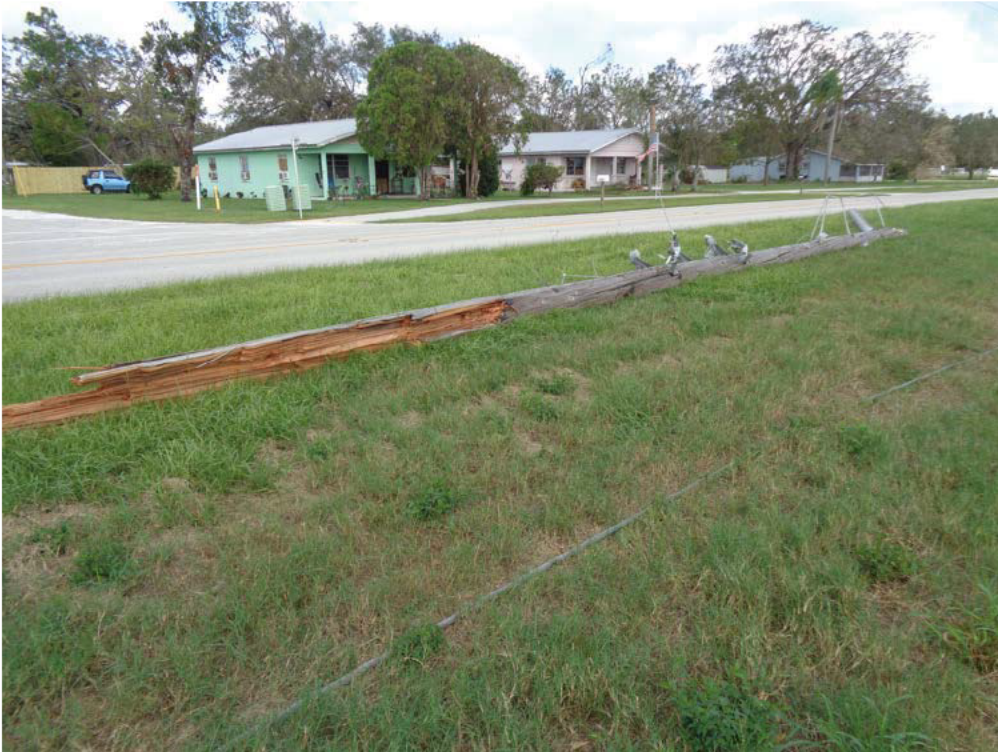
Failed wood pole AD-21. Looking northwest.
