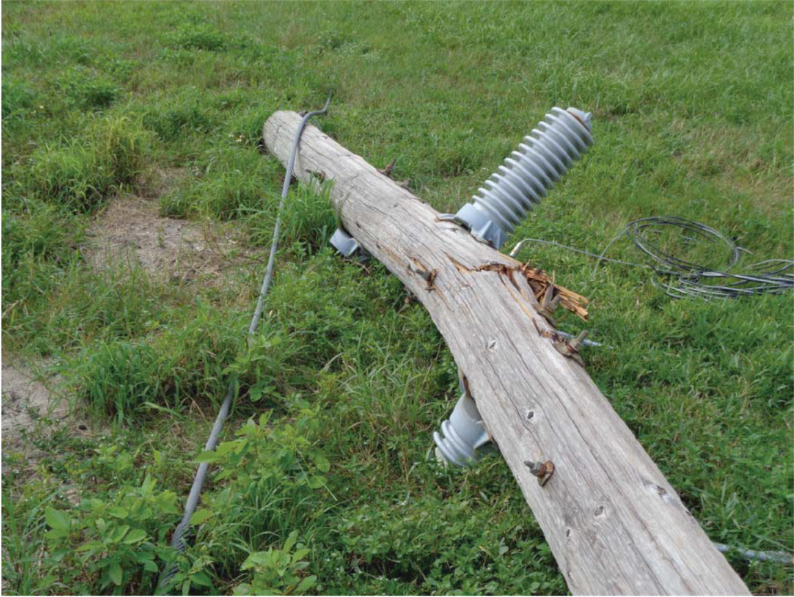
Wood pole AD-19 insulator damage and pole crack. Looking south.
