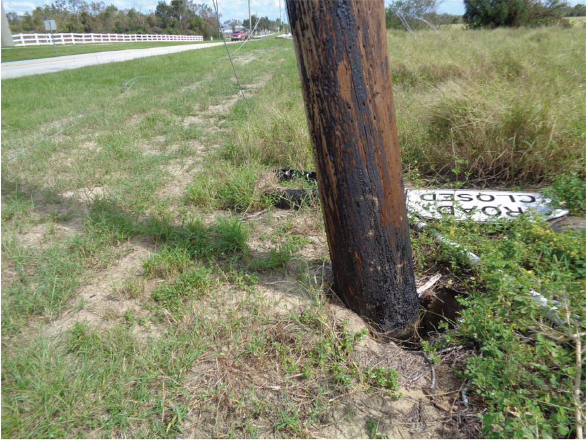
Wood pole AD-17 pole base. Looking north.
