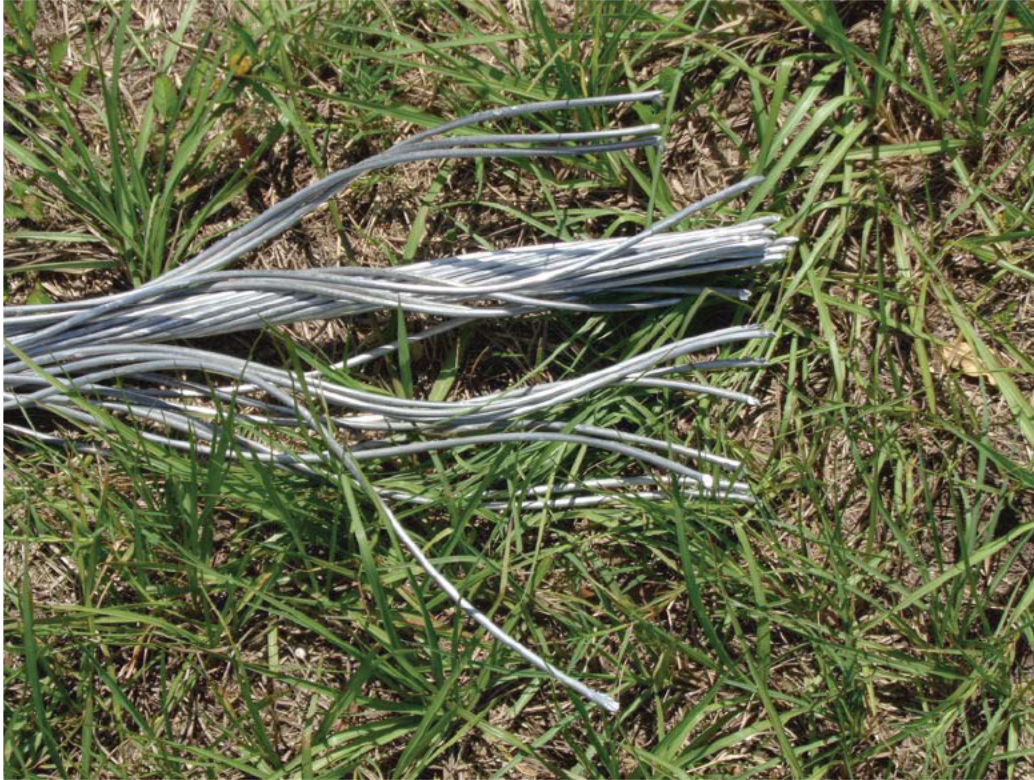
Broken wire, tensile failure. Between wood pole AD-17 and AD-18.
