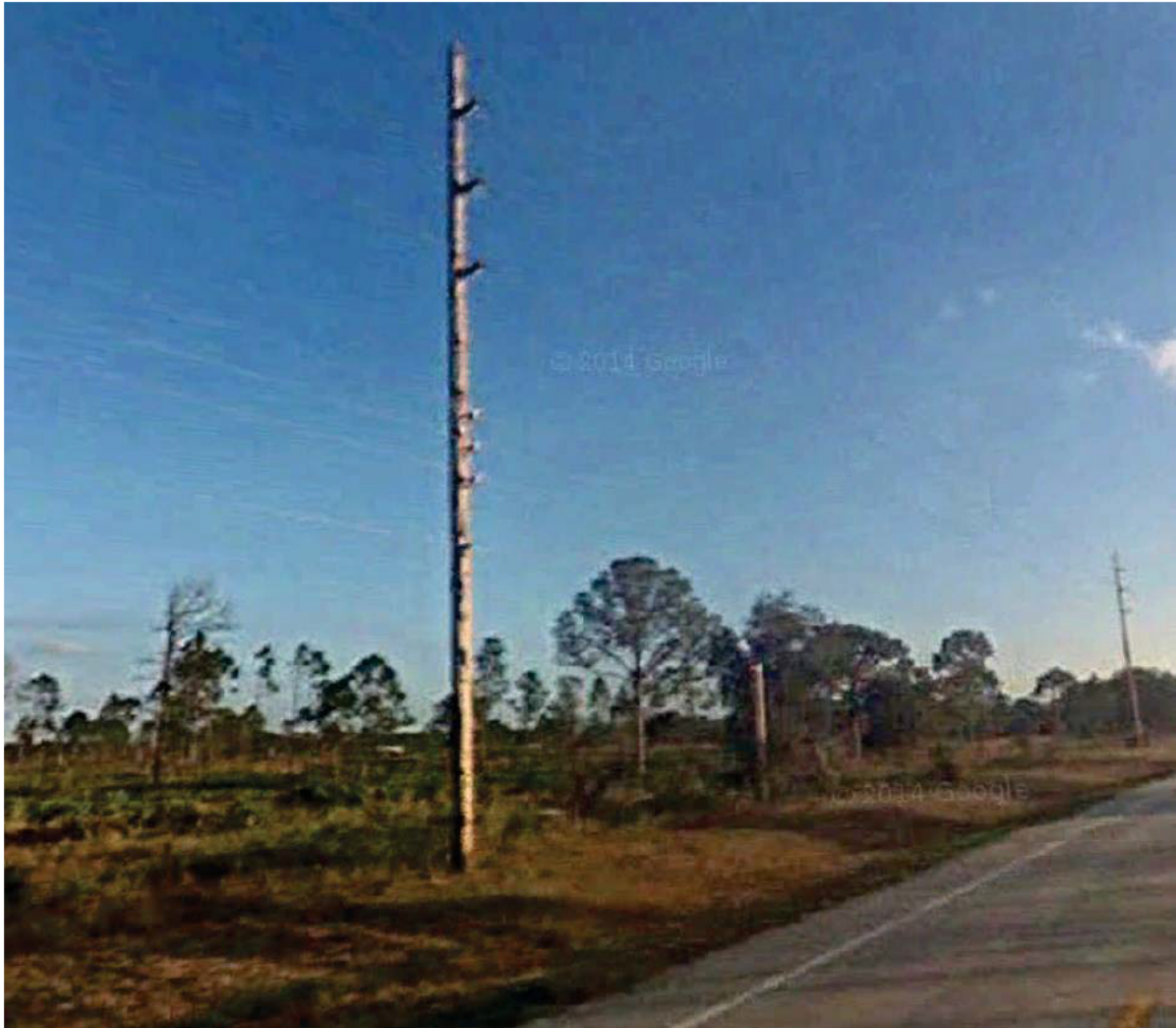
Figure 12: Failed pole ALP-208, looking southeast.
