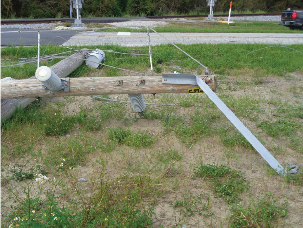
Wood pole AD-15 static mast. Looking west.
