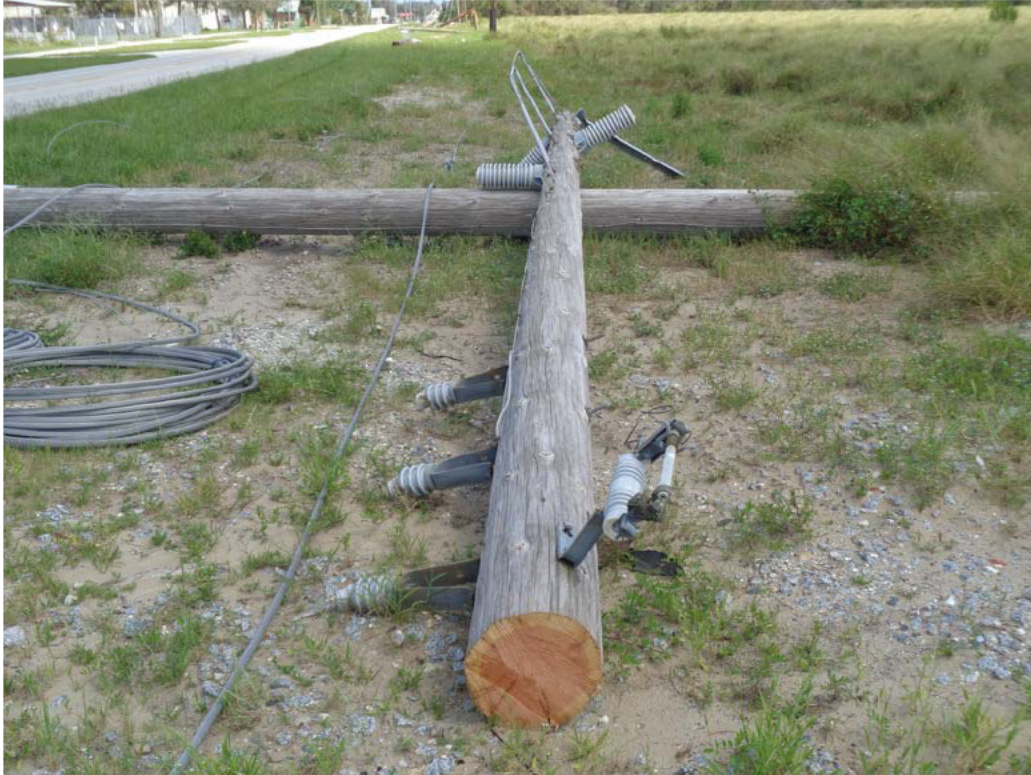
Failed wood pole AD-15. Pole was cut and relocated during the storm cleanup. Looking north.
