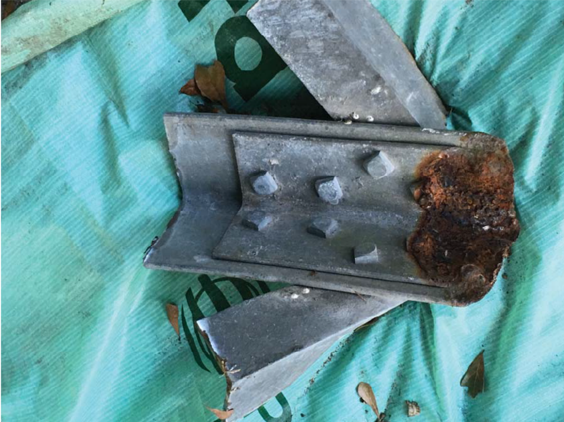
Tower HG-160 northeast leg corrosion.
