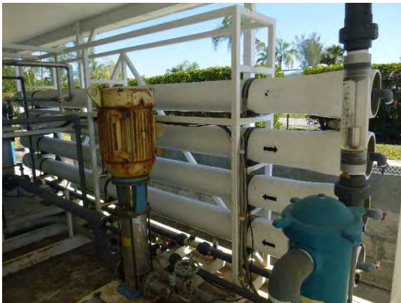
Photo 9: View of RO Trains and System.
