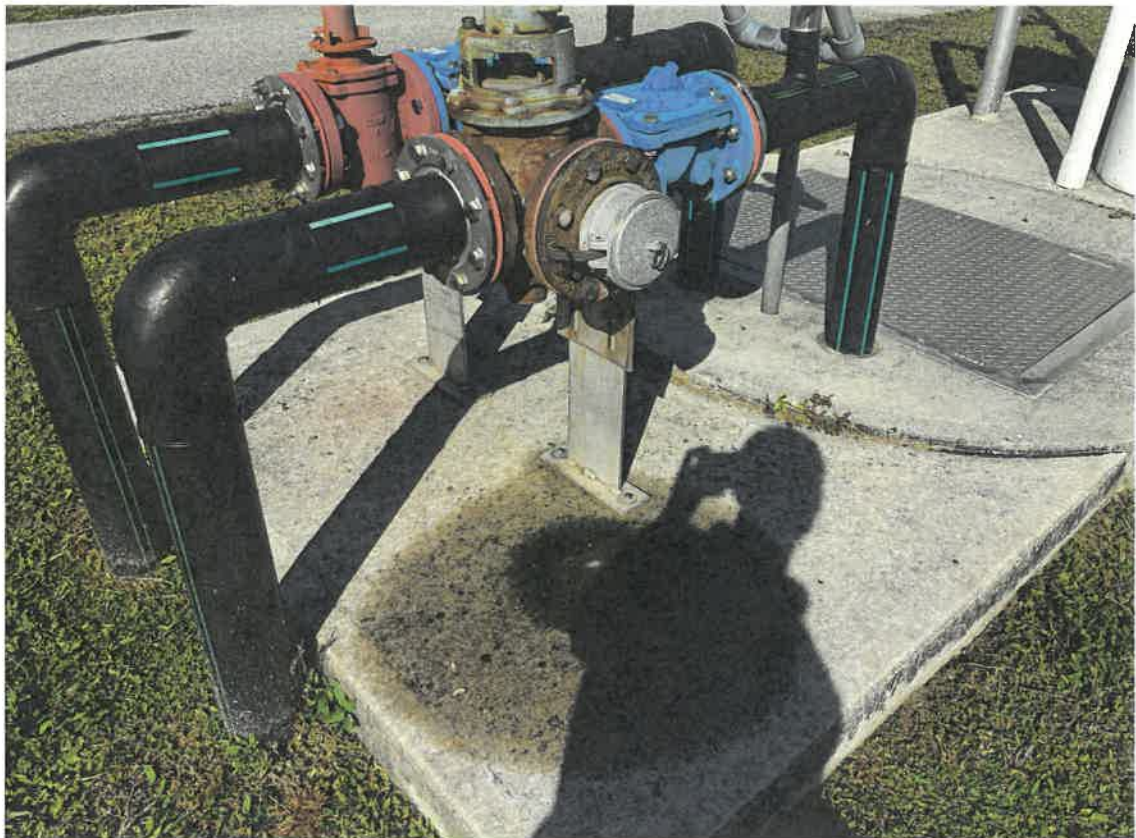
LIFT STATION SEAL LEAK
