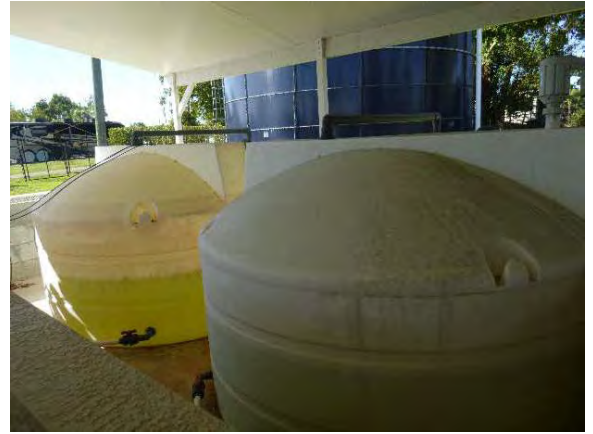
Photo 8: View of Chlorine Tanks.
