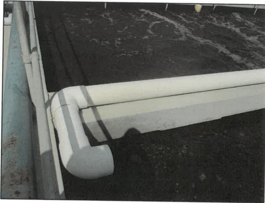
PHOTO 7: SOUTH PLANT INFLUENT PIPE
