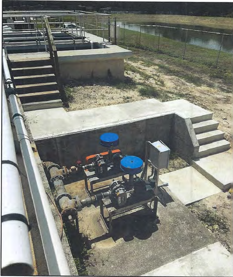
PHOTO 4 BLOWER UNITS FOR AIR SUPPLY TO PLANT 2
