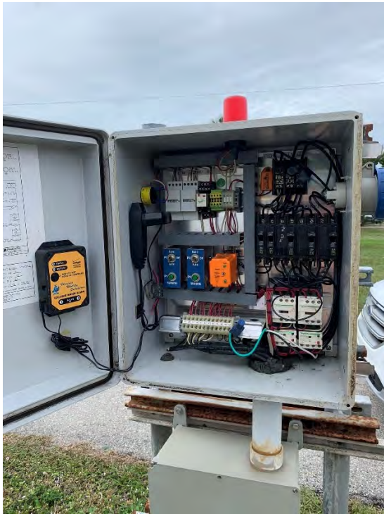
1. Lift Station #1 Control Panel
