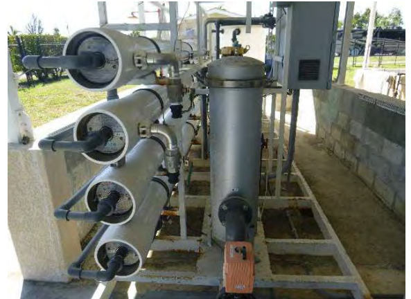
Photo 10: Continued view of RO trains.
