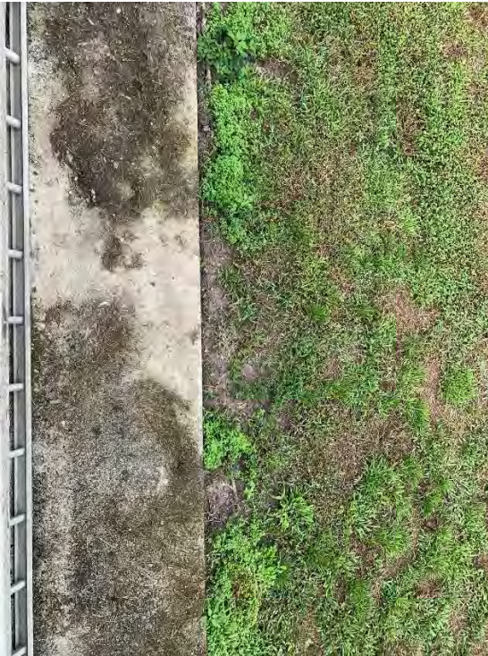
35. Signs of Headworks Overflow (Detritus)
