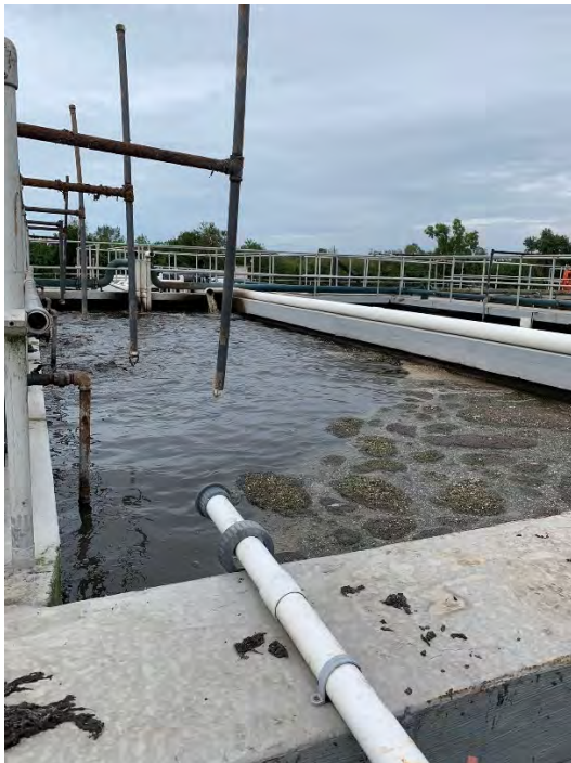
11. Aeration Basin and WAS Line
