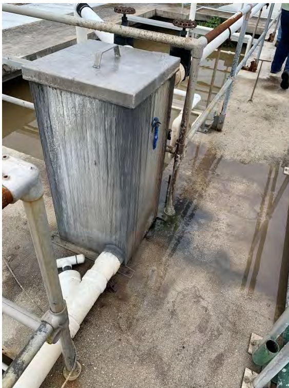
39. Severely Splashing Return Box
