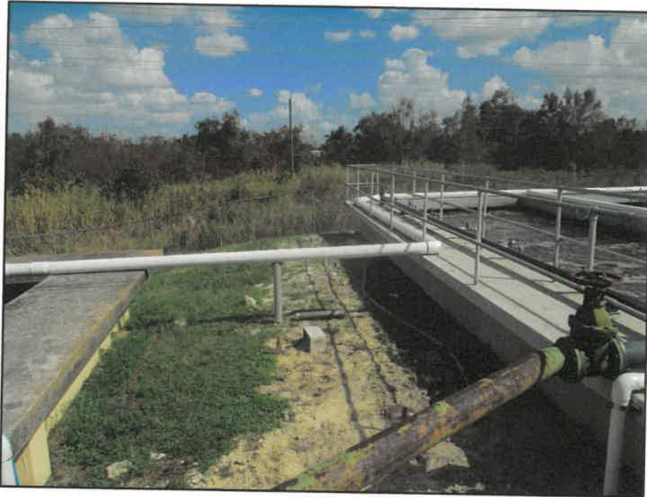
PHOTO 3: NORTH PLANT INFLUENT PIPING WITH SUPPORT
