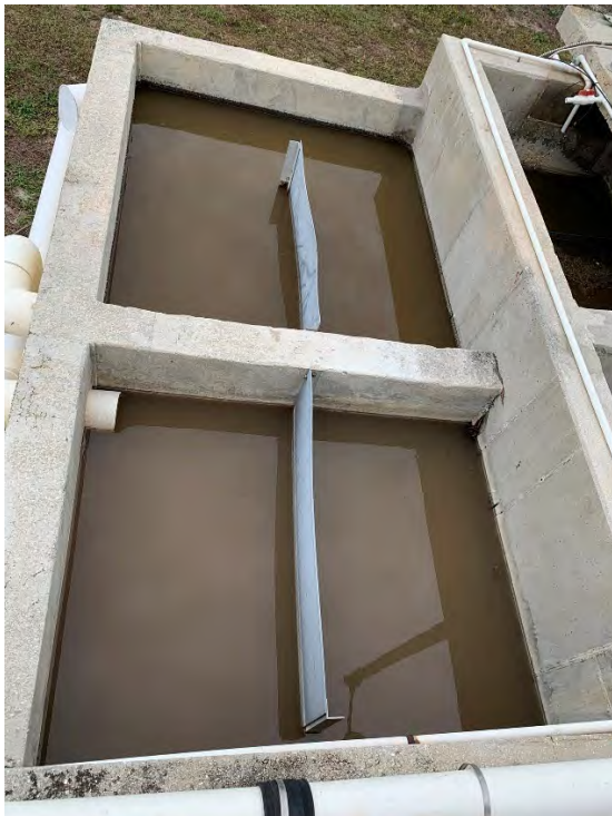
19. Chlorine Contact Chamber
