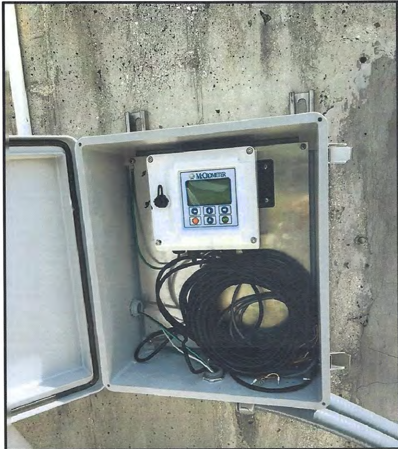
PHOTO 3 EFFLUENT FLOW METER OUTPUT CONTROL MONITOR
