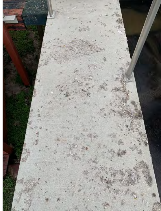
34. Signs of Headworks Overflow
