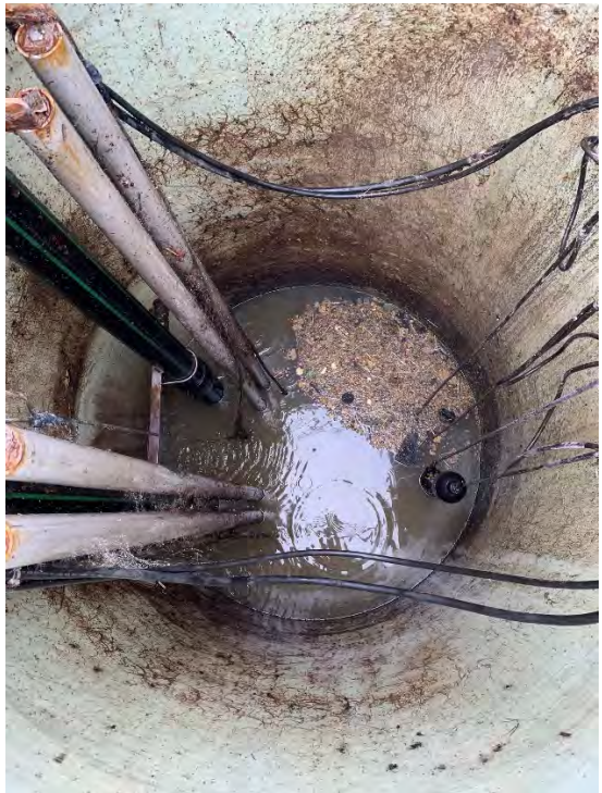
4. Lift Station #2 Wet Well
