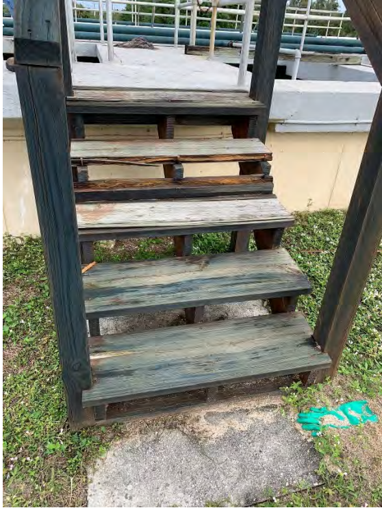
37. Steps with Broken Tread
