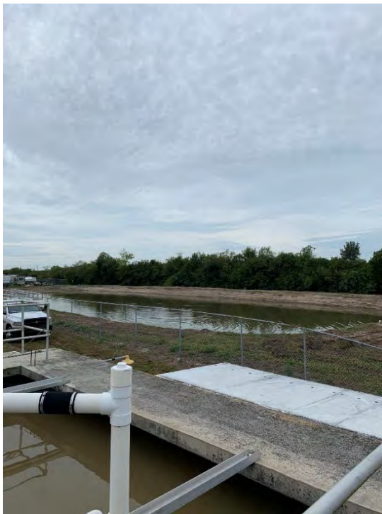
23. Rapid Infiltration Basin
