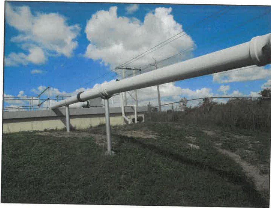
PHOTO 13: INFLUENT PIPE FROM SURGE TANK WITH SUPPORTS
