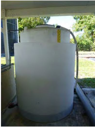
Photo 7: View of Ammonia Tank.
