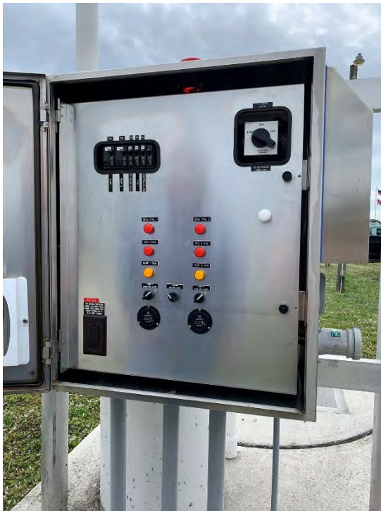
3. Lift Station #2 Control Panel
