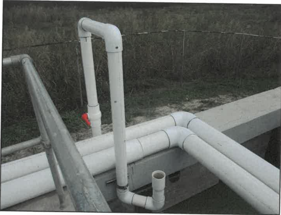
PHOTO 9: WAS PIPING AT DIGESTER
