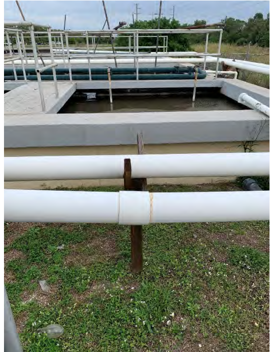
10. Sagging Influent Pipe
