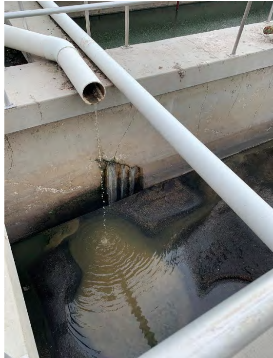
36. Leaking Crack between Digester and Surge
