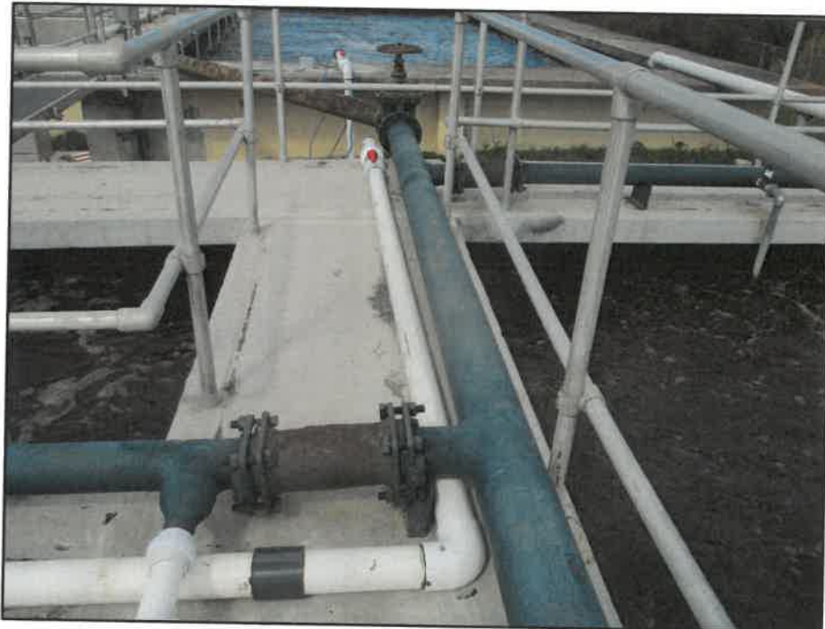
PHOTO 4: WAS PIPING FROM NORTH PLANT
