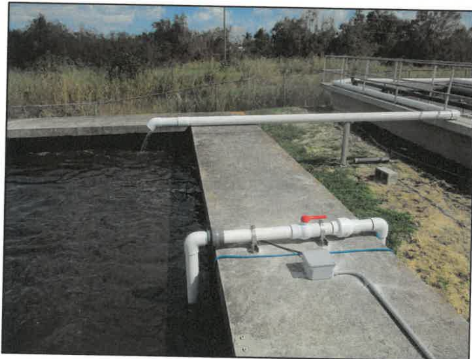
PHOTO 2: FOREGROUND WAS PIPING BACKGROUND NORTH PLANT INFLUENT PIPE
