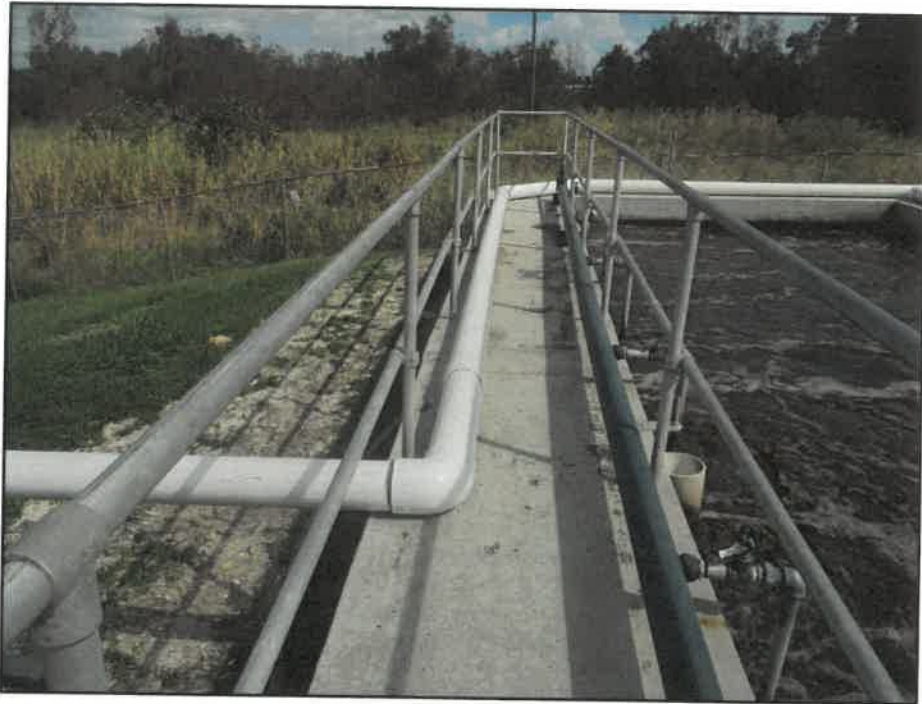
PHOTO 5: INFLUENT PIPING TO NORTH PLANT
