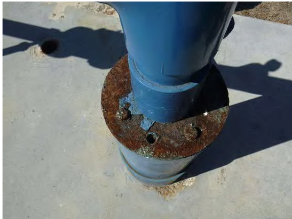
Photo 2: View of Well missing well vent.
