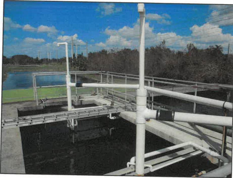
PHOTO 1: CLARIFIER RAS AIR LIFT PIPING NORTH PLANT
