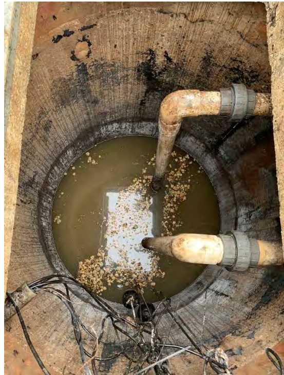
2. Lift Station #1 Wet Well
