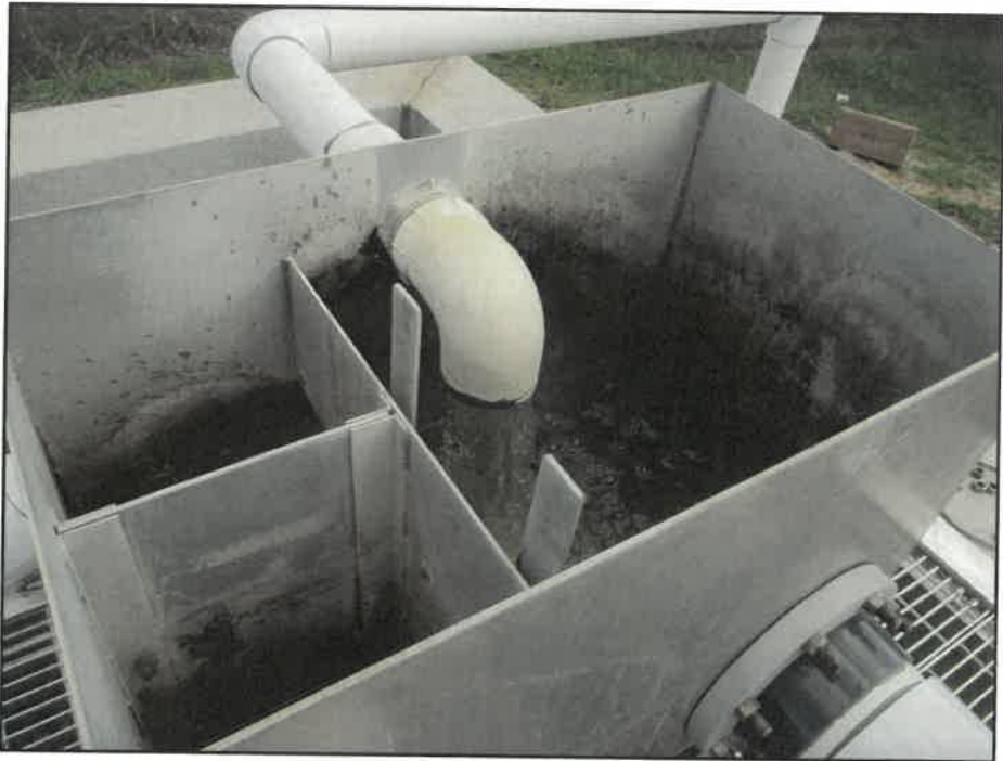
PHOTO 11: FLOW SPLITTER BOX
