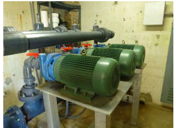
Photo 12: View of High Service Pumps.
