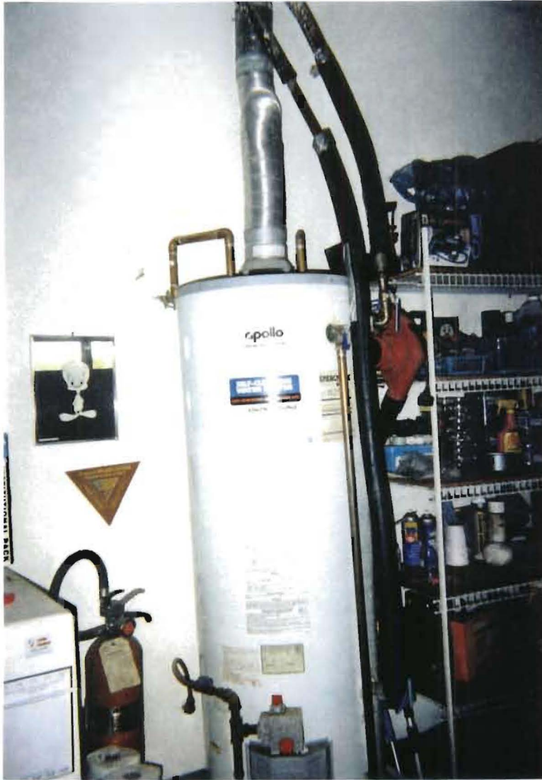
HOT WATER HEATER AT COOGAN RESIDENCE AT 1430 DAVENPORT DRIVE
