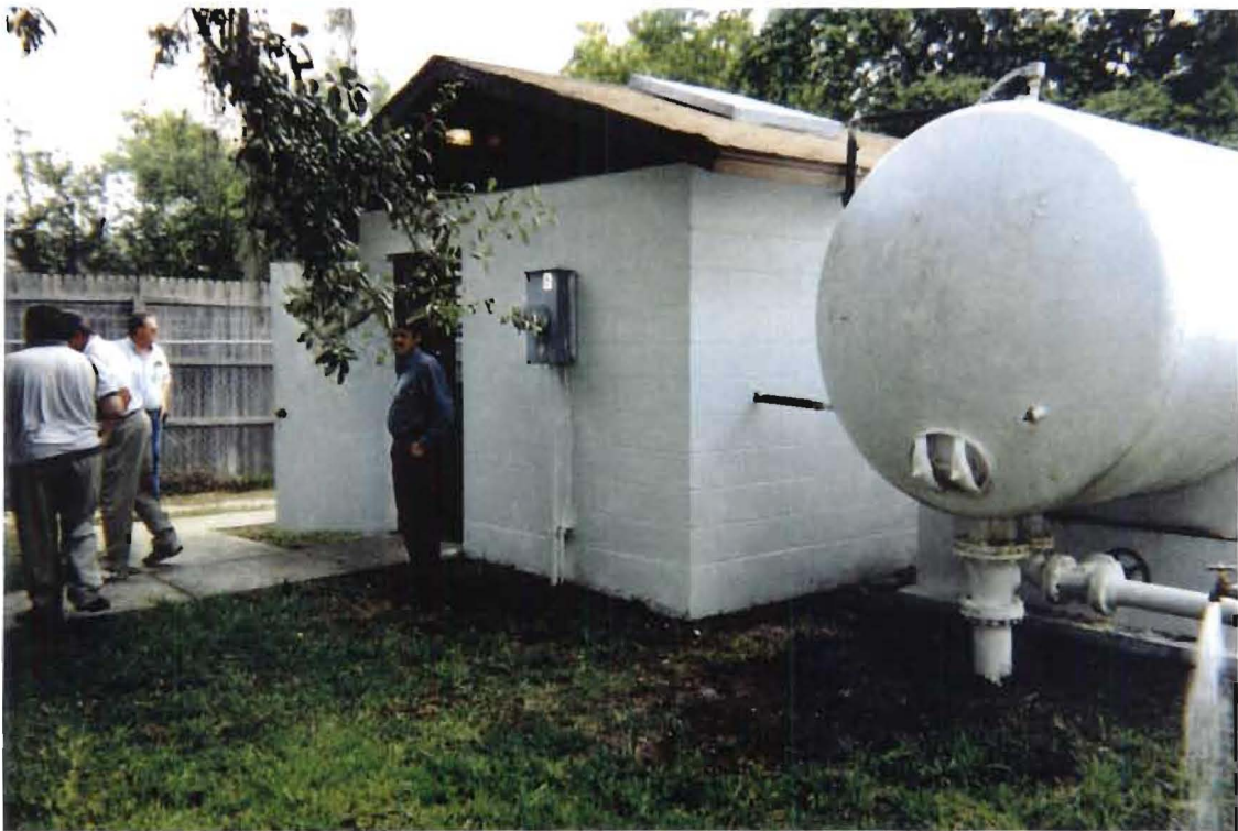
YARD VIEW OF WELL NO. 6
