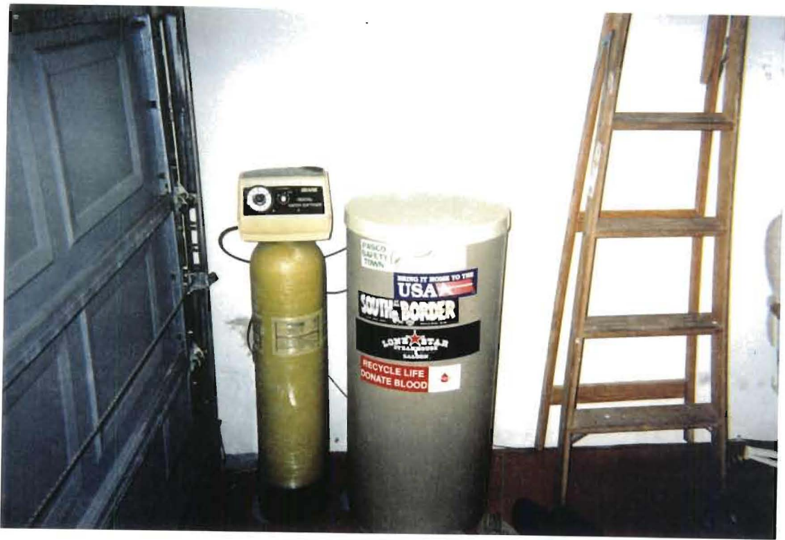
WATER SOFTENING UNIT AT COOGAN RESIDENCE
