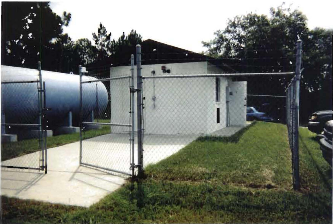
YARD VIEW OF WELL NO. 8
