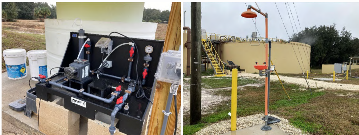
New variable chemical dosing pump (left) and emergency chemical shower and eyewash station (right)
