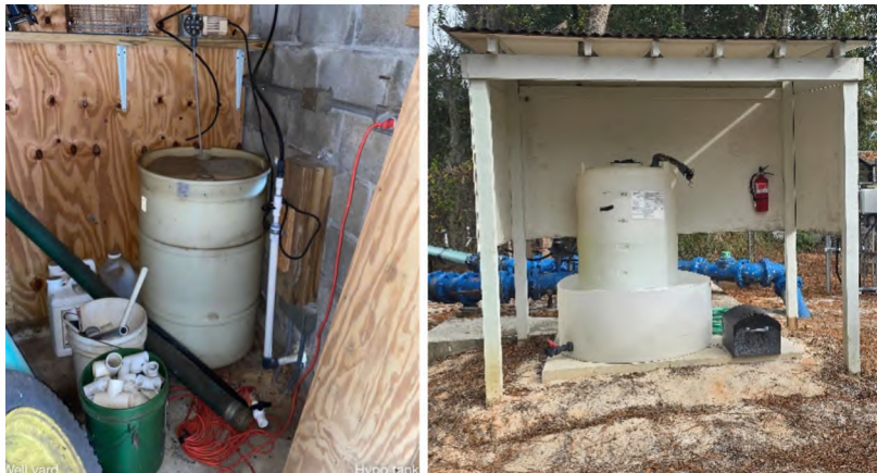
12 Disinfection system before (left) and after (right) improvement.
