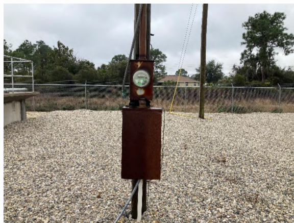
Extremely corroded existing 200 amp power supply.
