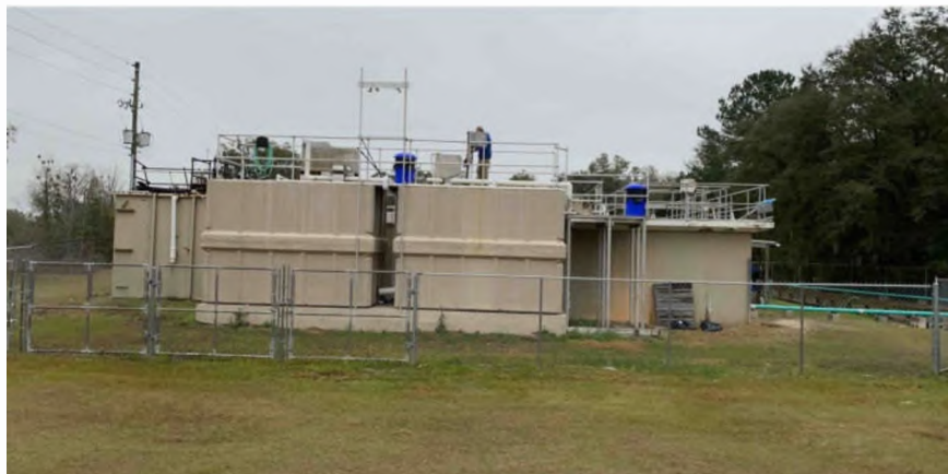
Ground level overview photo of Landfair WWTF at acquisition.
