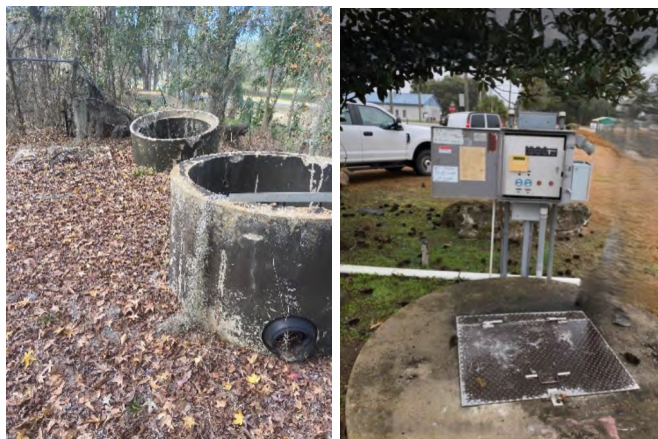
Damaged unused manhole rings, trash, and vegetation overgrowth at Tradewinds lift station site, including vegetation causing fence damage (left). Tradewinds lift station lacking fencing (right).
