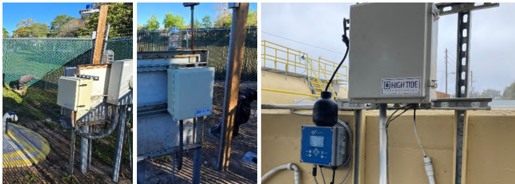
Examples of new remote monitoring equipment installed at the lift stations (left and center) and the treatment plant (right).
