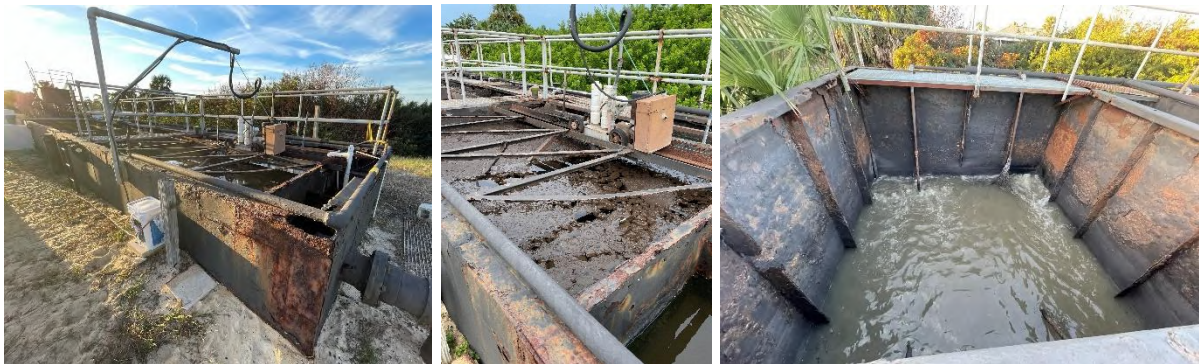
7 Examples of steel tanks and equipment deterioration at closing and examples of the numerous poorly installed 8 welded patches on the tanks. 9 10
