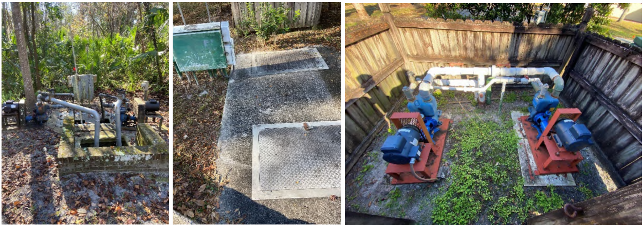
9 10 Lift Stations 1 (left), 2 (center), and 3 (right).
