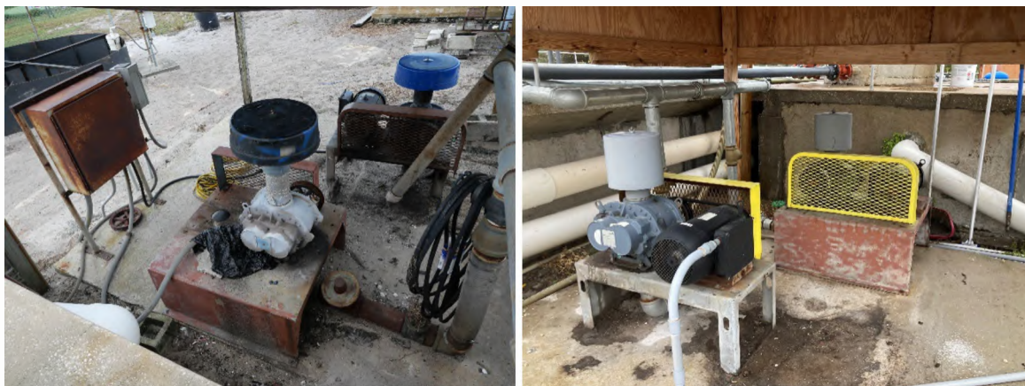
7 8 Blowers before (left) and after (right) improvements.
