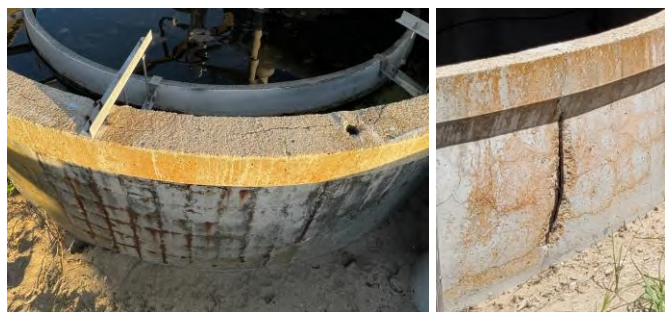
11 Examples of cracking and exposed rebar in concrete tanks. 12
