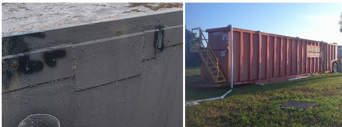
Example of patching leaks in steel tanks at North Peninsula (left) Temporary tank in place since concrete tank failure (right).
