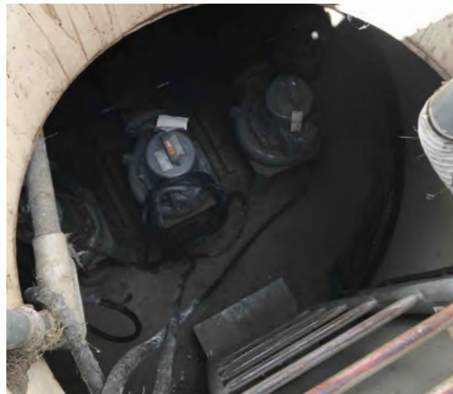
Lift station 2 dry well basin
