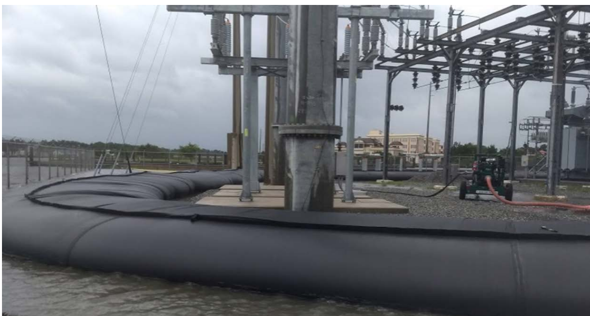
AquaDam held back storm surge and an interior pump kept rain from accumulating
