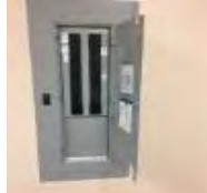
Common Circuit Breaker Panel
