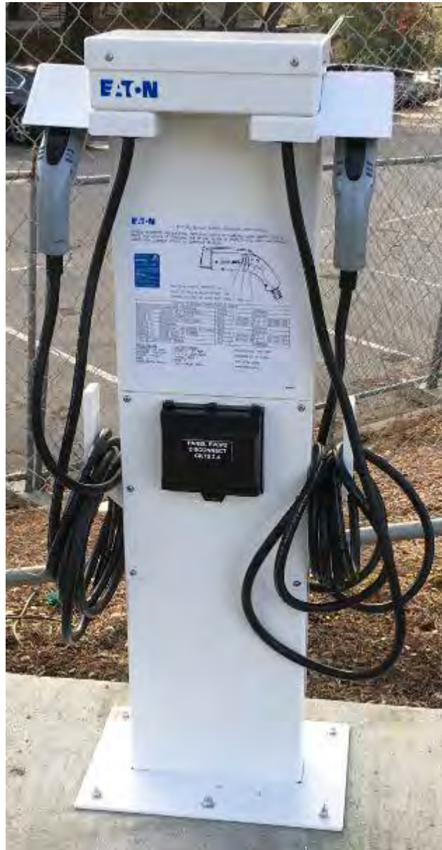
Figure 23 Dual Port EV-EMCB Charging Station Installed in Palo Alto, CA.
