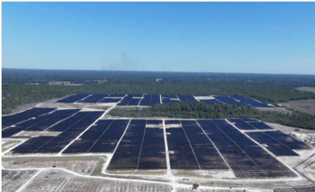
FIGURE 3.3 Half Moon Solar Power Plant
