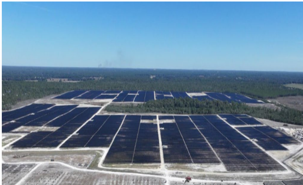
FIGURE 3.3 Half Moon Solar Power Plant
