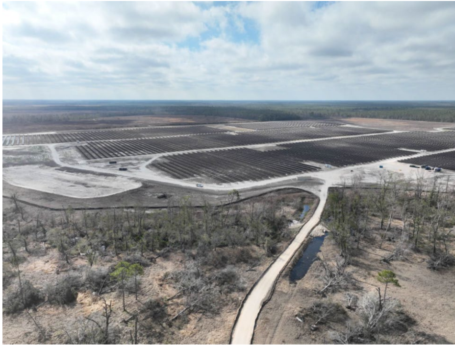
FIGURE 3.2 Sundance Solar Power Plant
